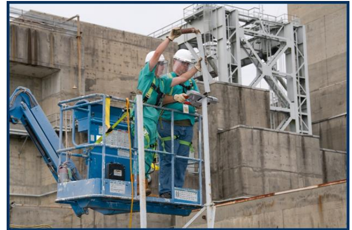
R Reactor Recovery Act workers at SRS saw fixture piping as D&D work begins.
