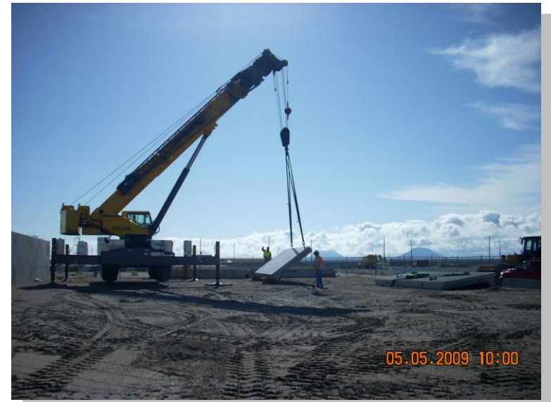
The HIC enclosure was the first decontamination and decommissioning project completed under the Recovery Act.
