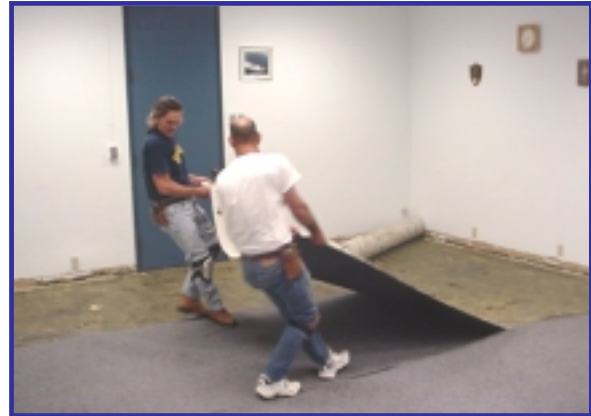
Manual removal of carpet in a large space took two workers 160 hours.
