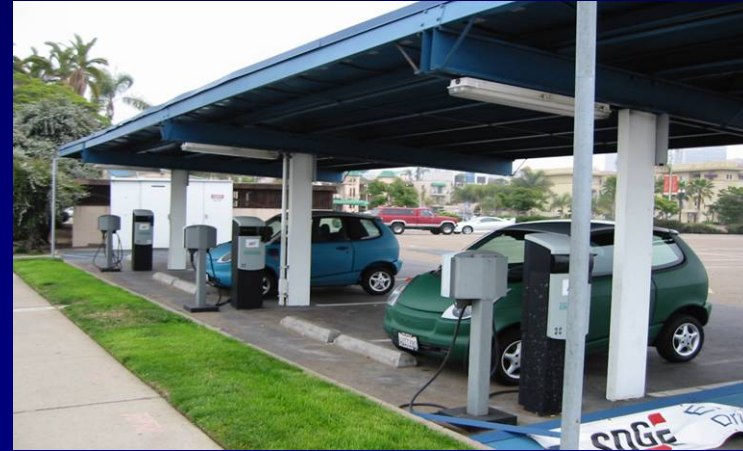
10 kW EV Charging Station
