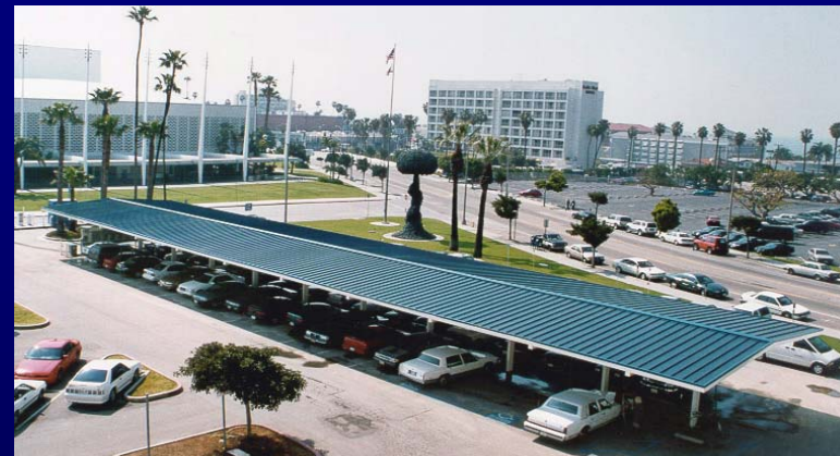
30 kW Parking Shade Structure
