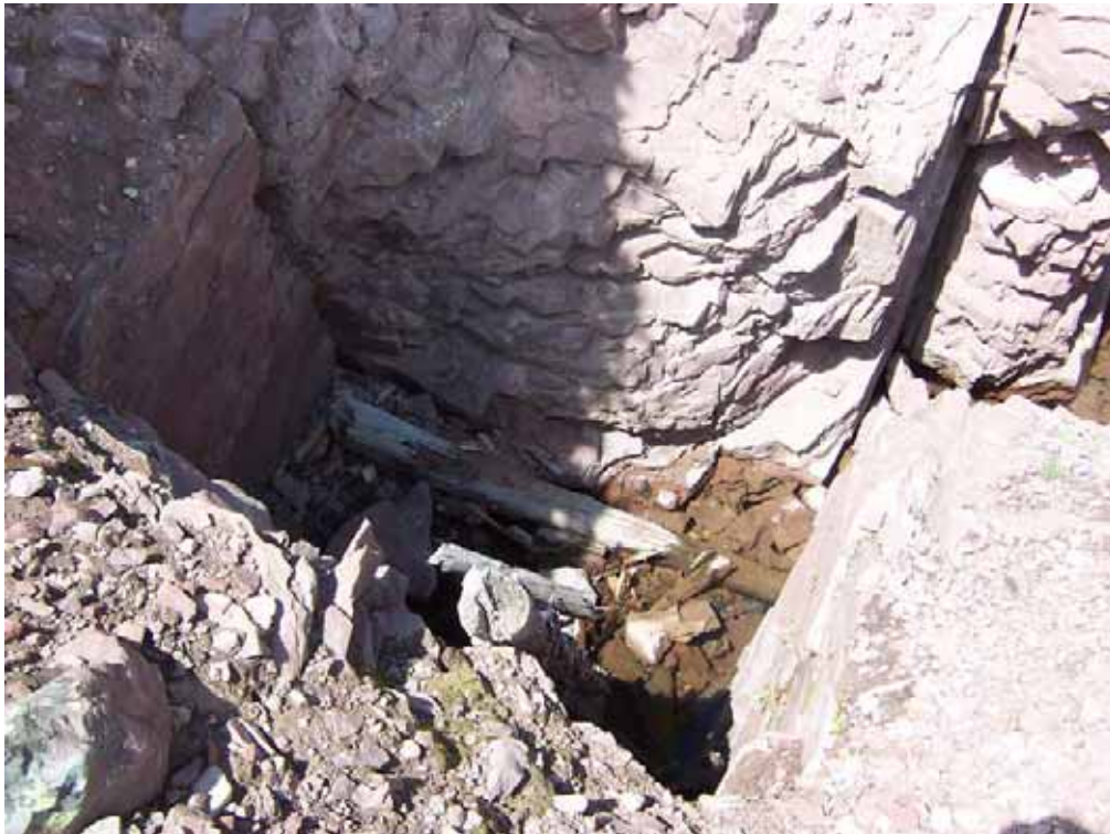
Figure 8: Looking down into inlet hole, note debris clogging inlet.
