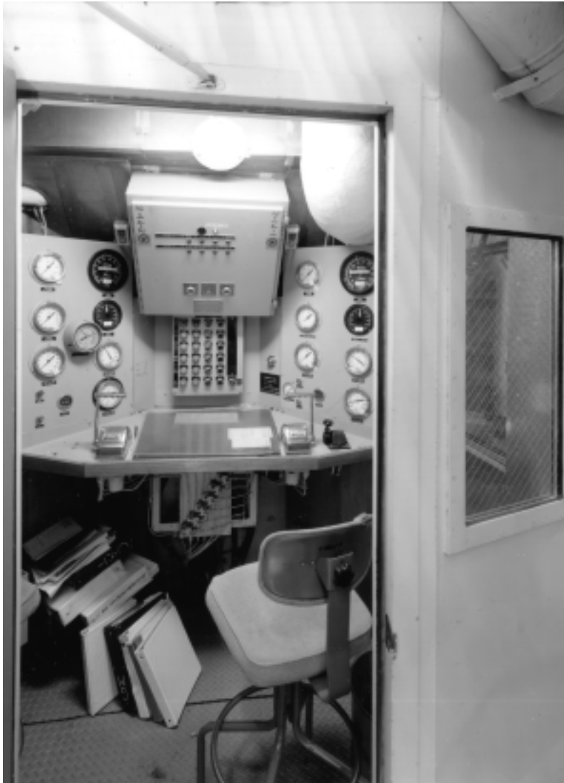
White Sage's enclosed control room (1999 HAER photo).
