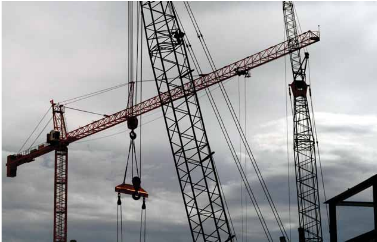
FESTIVAL OF THE CRANES — Construction cranes, including a 190-foot giant, tower over the MESA construction site on the east side of Tech Area 1. The cranes, brought in by general contractor Hensel-Phelps for work on the MESA MicroLab facility, are the most visible sign yet that the MESA project is moving full speed ahead. The multi-building MESA complex, scheduled to be completed in 2007 with a price tag of more than $450 million, is the largest building project in Sandia's history. (Photo by Bill Murphy)
