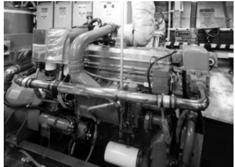
Ship's generator aboard Sundew. HABS/HAER photo by Jet Lowe.
