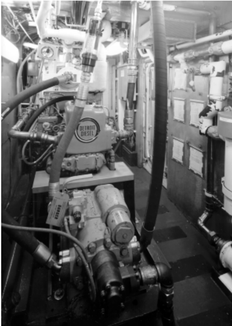
Diesel engine that powers the hydraulics for boom on Bramble. HABS/HAER photo by Jet Lowe.
