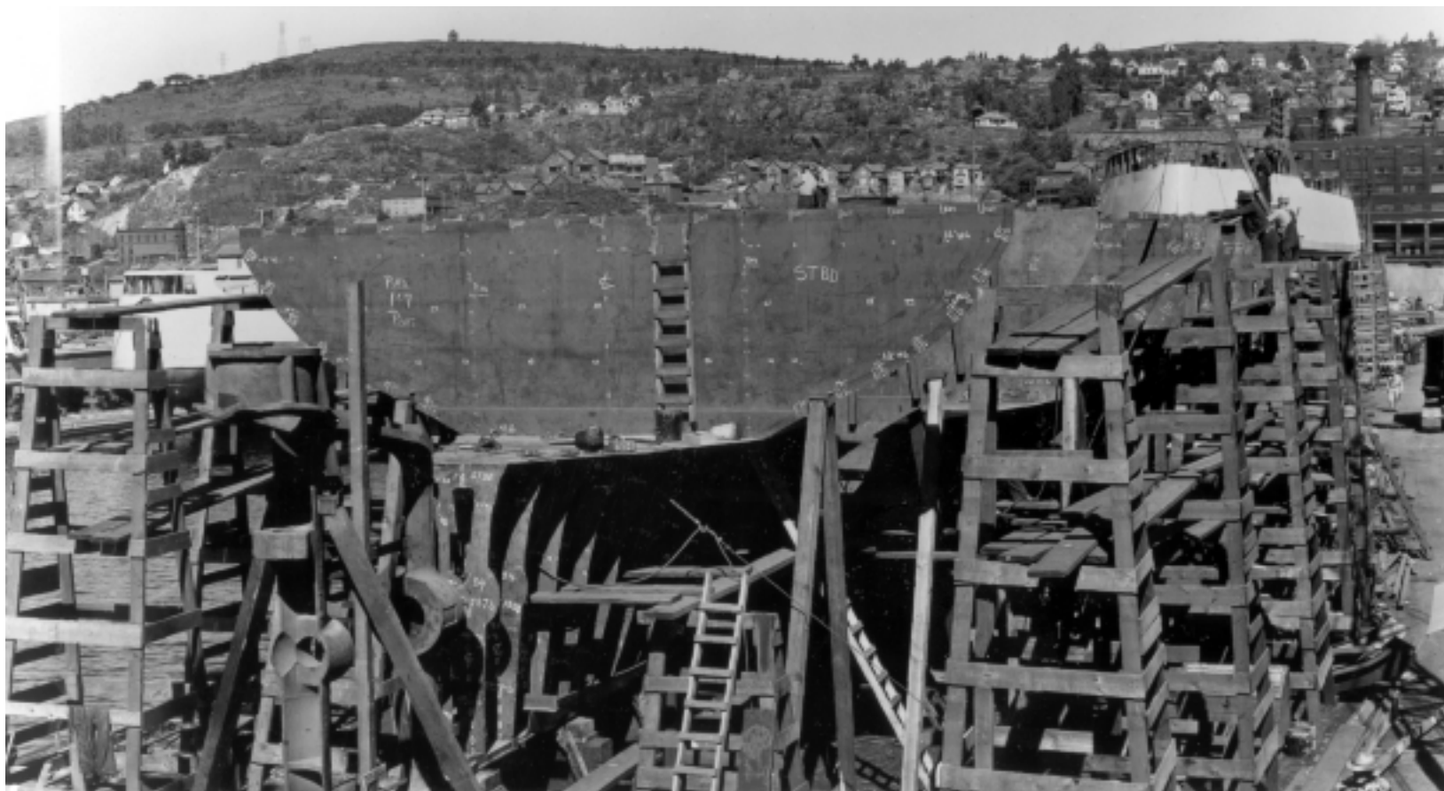
Two 180s at different stages of construction. Note the series of bulkheads that subdivide the vessel's hull into several smaller compartments. Visible in the left foreground is the assembly that will eventually hold the rudder as well as the collar through which the propeller shaft will pass.
