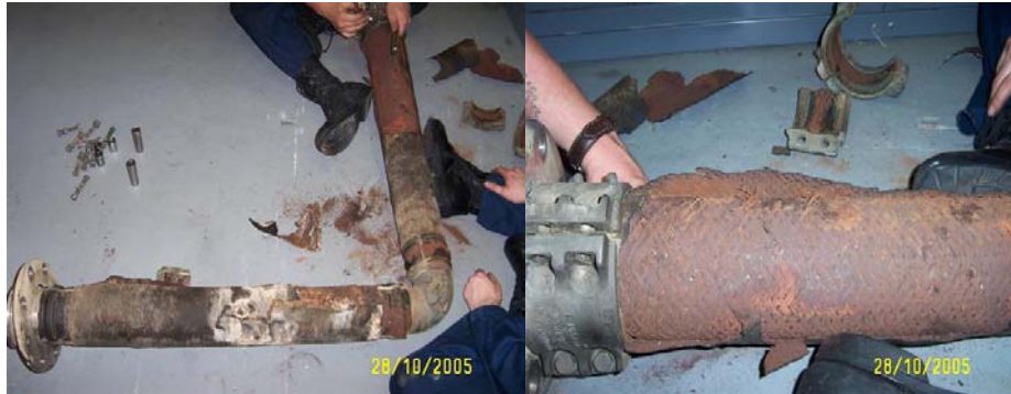
Jacket water hose
