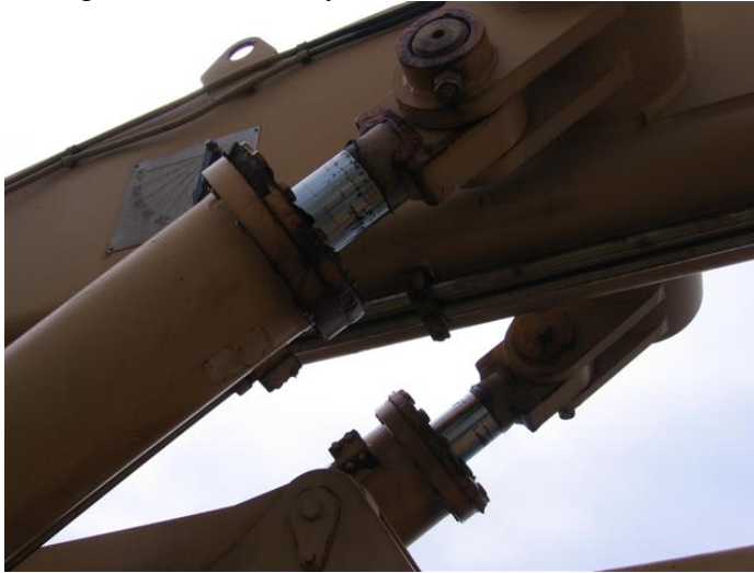
Main boom cylinders corroded and leaking
