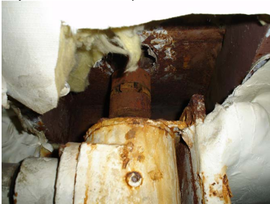
Anchor Windlass corrosion
