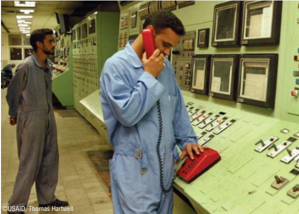
Iraqi engineers monitor controls at the Baghdad South power plant. IRRF funds are helping to repair Iraq's nationwide electrical system.
