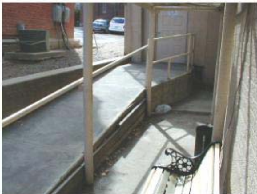
Left: Before Renovations (Note slope is out of compliance with ADA)
