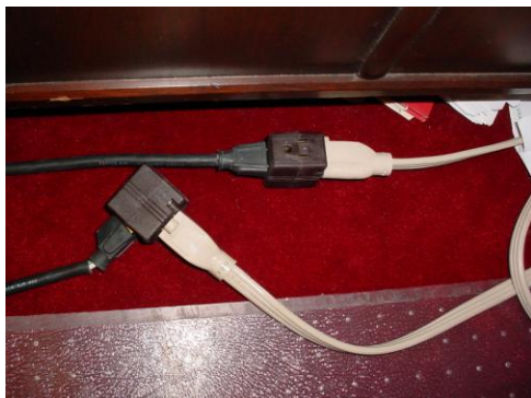
Picture 3 Extension Cords and Cube Tabs in Use
