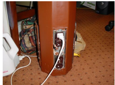
Picture 2 Faceplate missing from outlets
