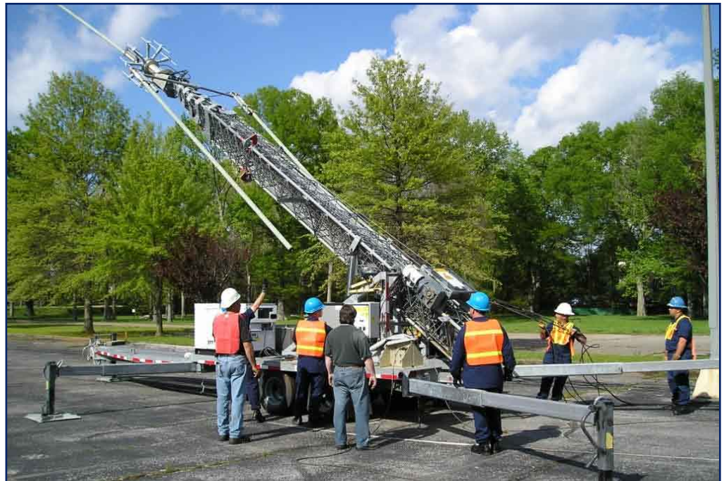
Communications Area Master Station Atlantic team members test a 127-foot portable tower equipped with Rescue 21 antennas as part of a recent training exercise in Huntsville, Ala. U.S. Coast Guard photo by Lt. Mark E. Moriarty
