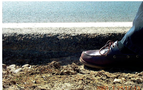
Sharp, steep pavement edge drop-offs can contribute to crashes.
