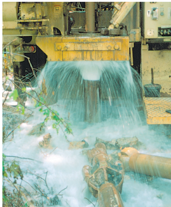
Discharge from air-lifting ground water from a well after penetrating water-bearing fracture zones
