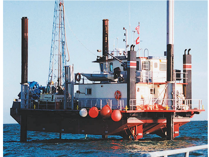
U.S. Army Corps of Engineers jack-up barge used as a platform for drilling offshore test borings near Hilton Head Island
