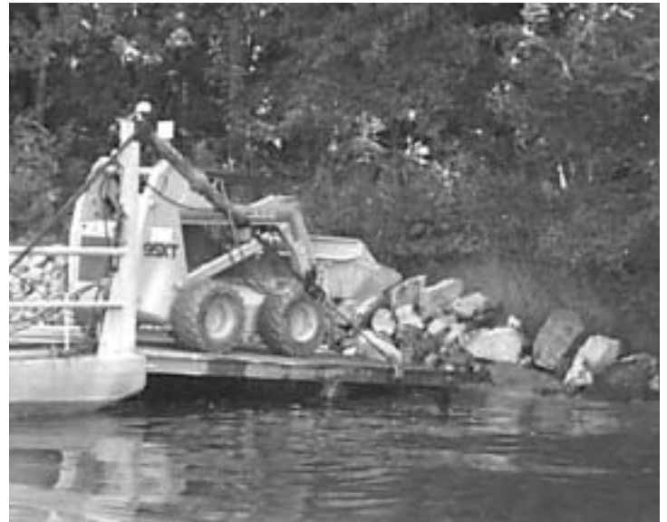
Consistent with federal regulations, TVA has implemented a program to conserve and protect significant archaeological sites along the riverbank through the placement of riprap—a permanent cover of rocks often used to stabilize shoreline. The riprap, which is delivered by barge, is carefully placed over the undisturbed site to protect it from erosion and looting.
