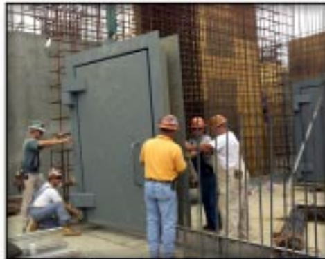
Bertha is used to lift and place large items such as this steel vault door for the Target Building.
