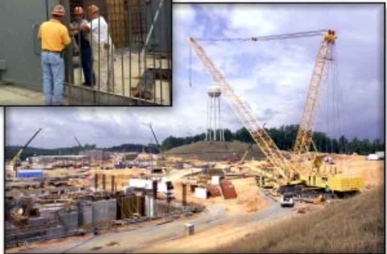
"Big Bertha" at the SNS site. This crane, one of the largest in the region, was given to the project by Lawrence Livermore National Laboratory, where it was known as "Manny Ringer."
