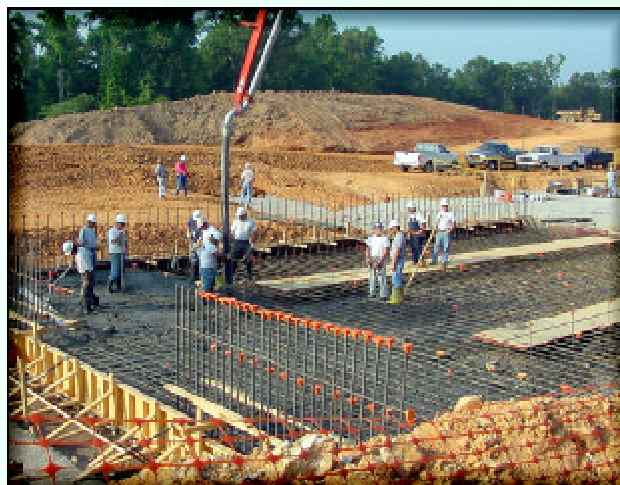
The first 200 cubic yards of concrete poured at SNS in June 2001 was for the front-end building.
