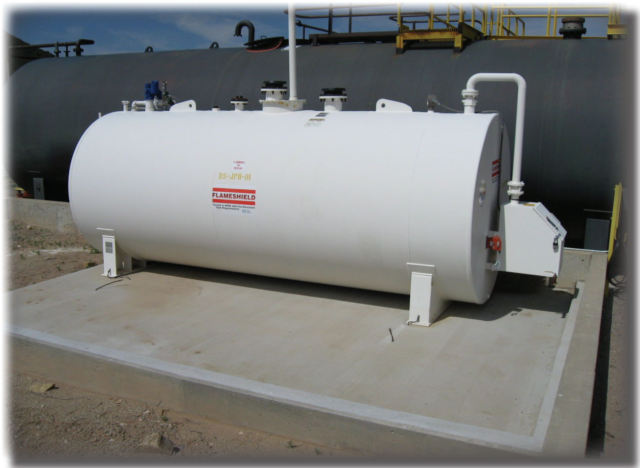
Aboveground Storage Tank
