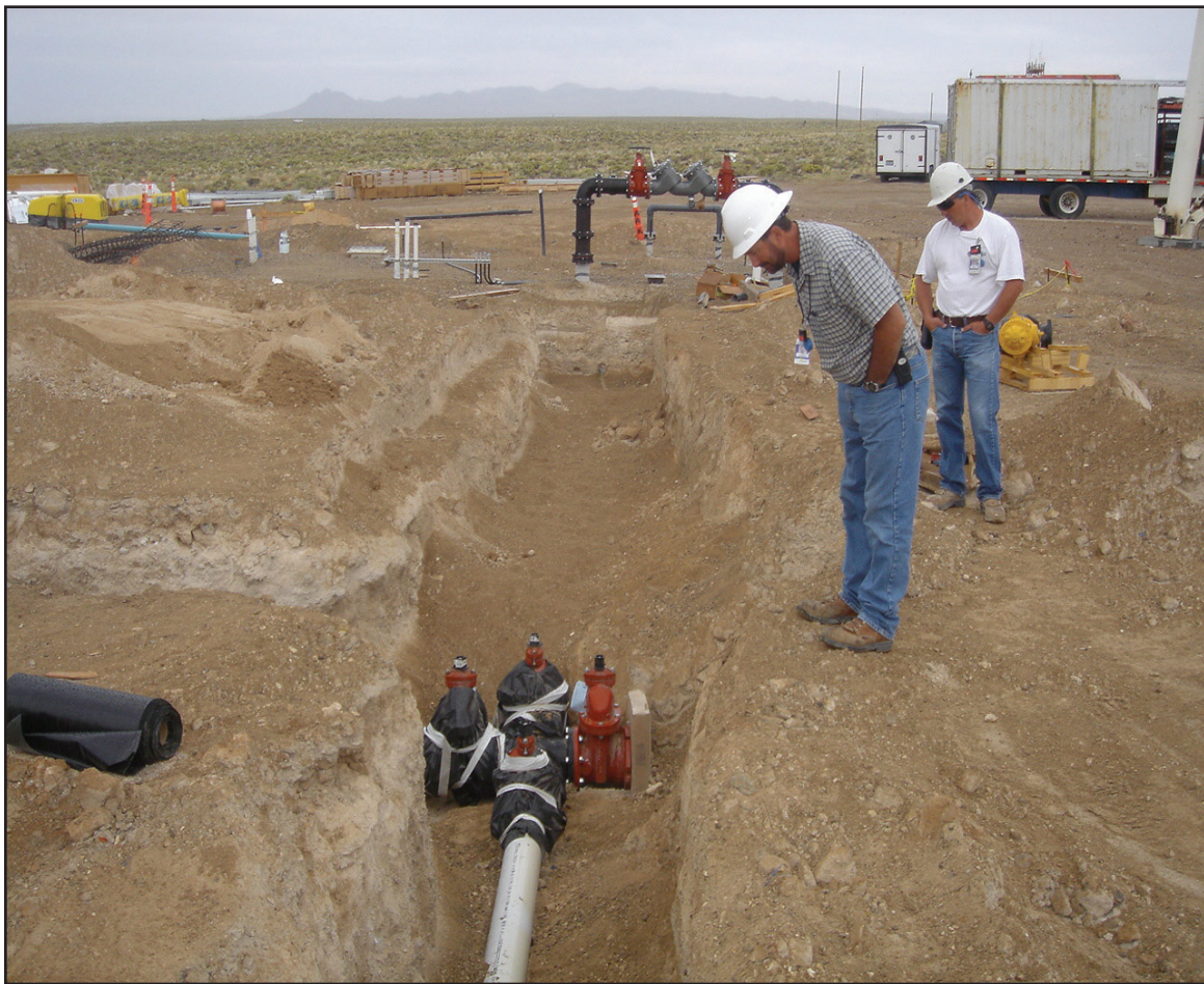
Workers inspecting the main distribution valves under the elevated water storage tower as part of the Water Distribution System Replacement Project.
