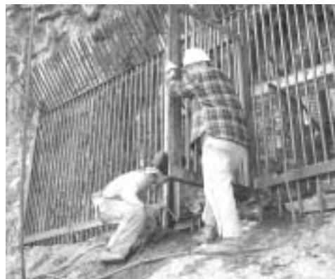
TVA has an active cave-gating program designed to prevent bats from being disturbed by human activity. This newly constructed gate at the entrance of Norris Dam Cave will help protect a colony of about 4,000 gray bats.
