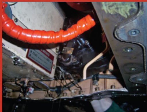
AMAD bay with white generator (normal) and black AMAD connected to the bulkhead (supposed to be white as well).
