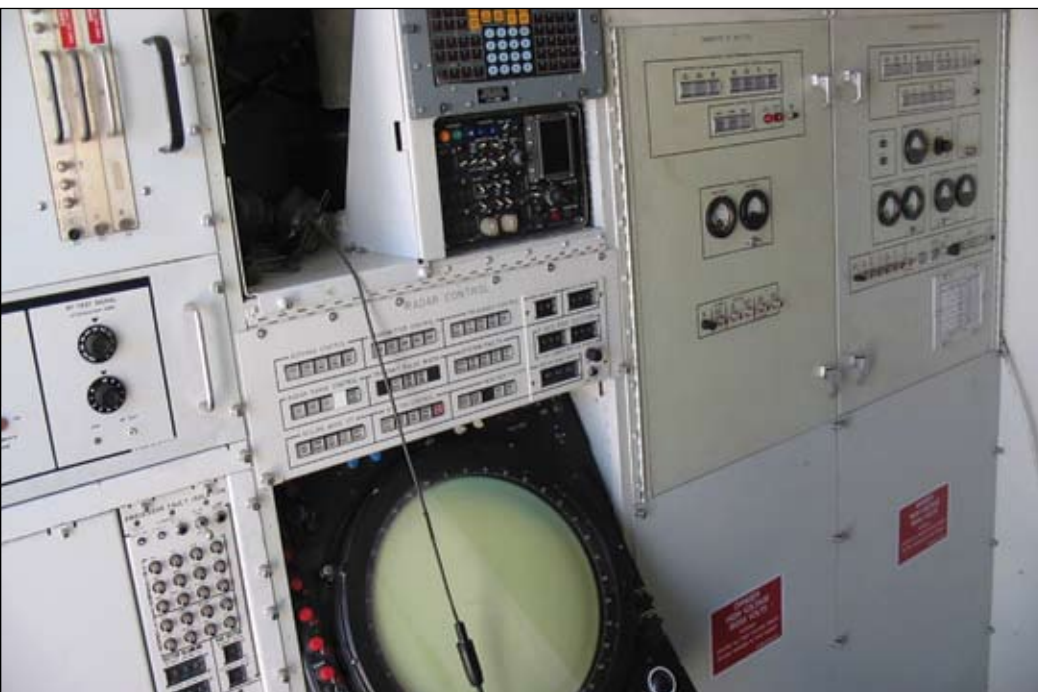
⤴ Switch board to the radar system is quite complex and requires strict adherence to procedures.
