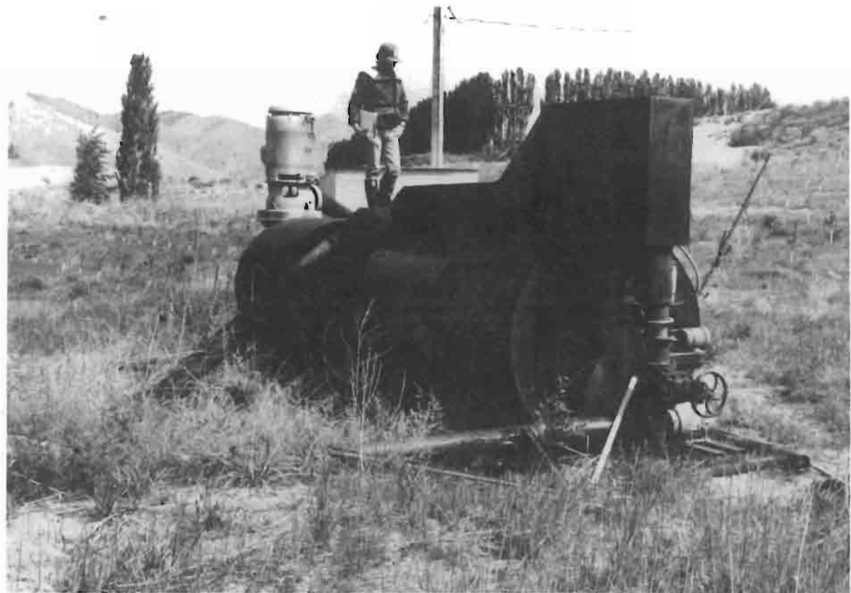
Figure 22.—Views of a typical small water withdrawal and screen system used along the upper Columbia River: a simple pump and intake line incorporated with an additional debris and weed seed straining device.
