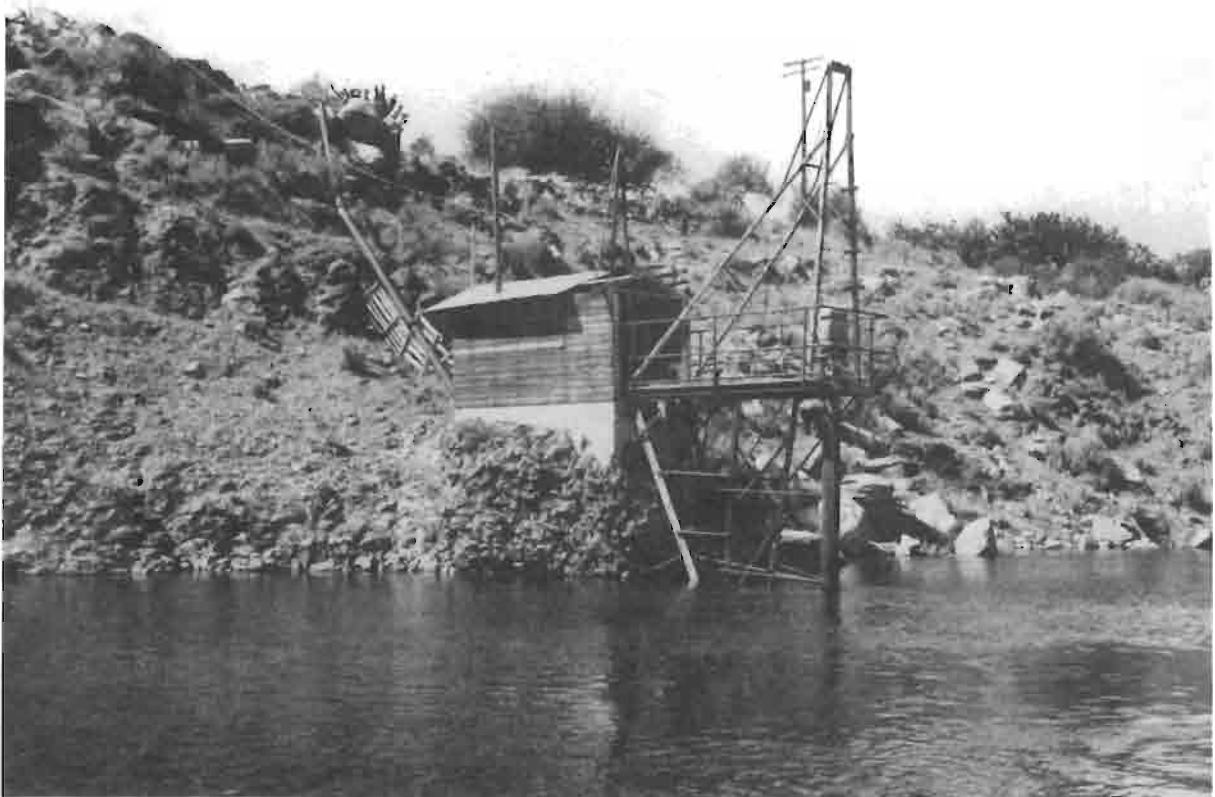
Figure 20.—Views of typical small pump installations throughout the study area. Note single intake line extending to a depth below the low water elevation.
