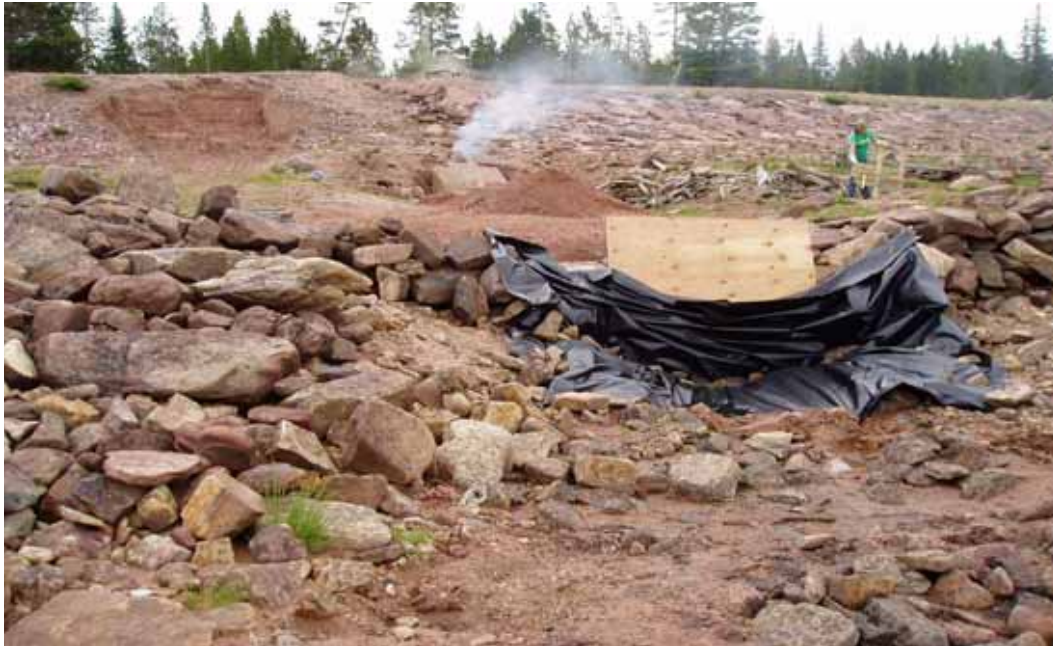
Figure 4 - The SCA used heat from burning logs removed from the shoreline to crack the vault and then break-up the materials with hand tools. Note start of excavation in the dam's embankment material. Riprap was stockpiled on both sides of the inlet channel for later use.
