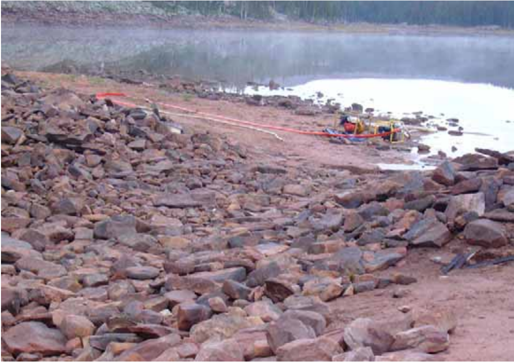
Figure 28 - View of finished upstream inlet channel graded and lined with rip rap.
