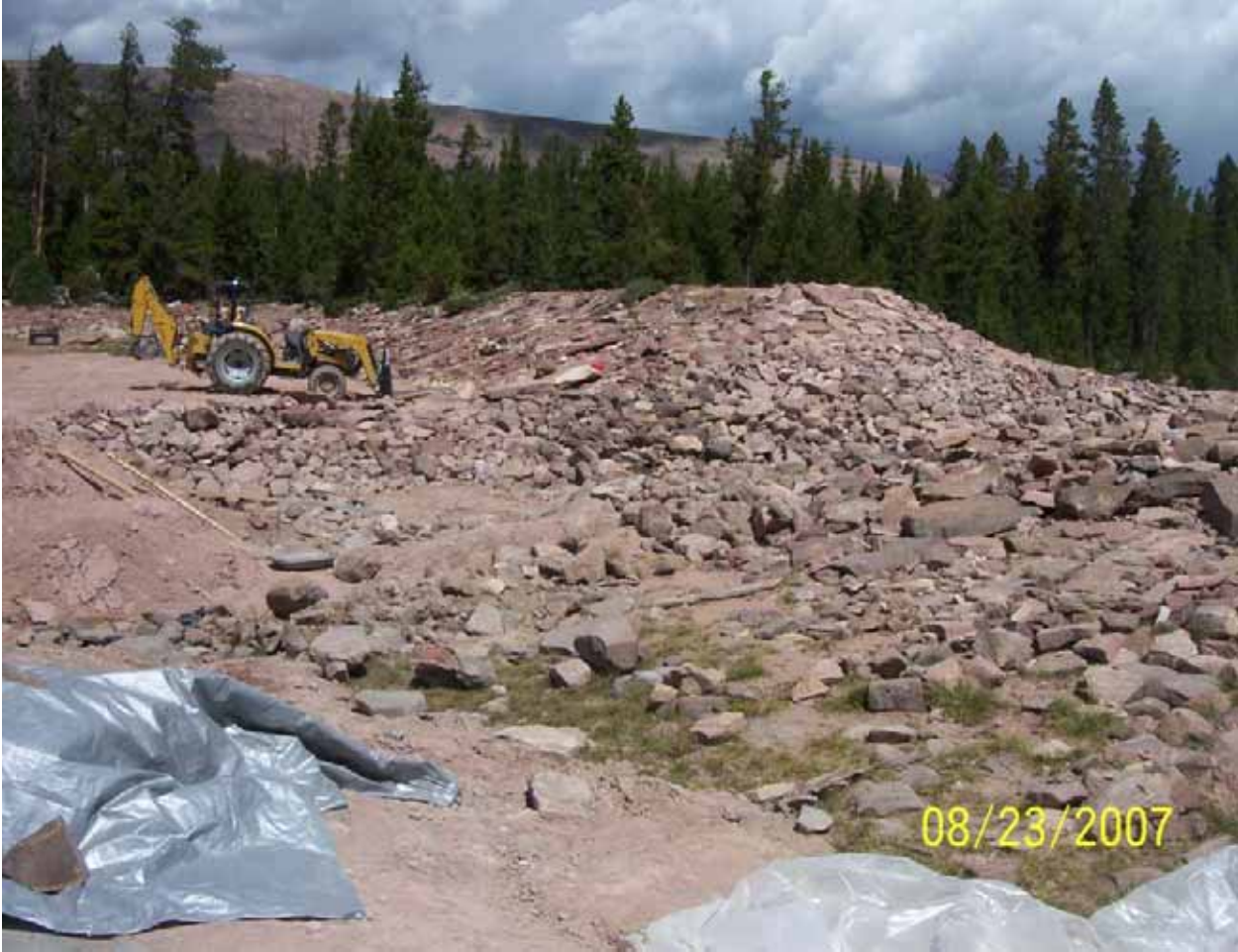
Figure 24 - View of dam site during construction as breach and inlet lining is progressing.
