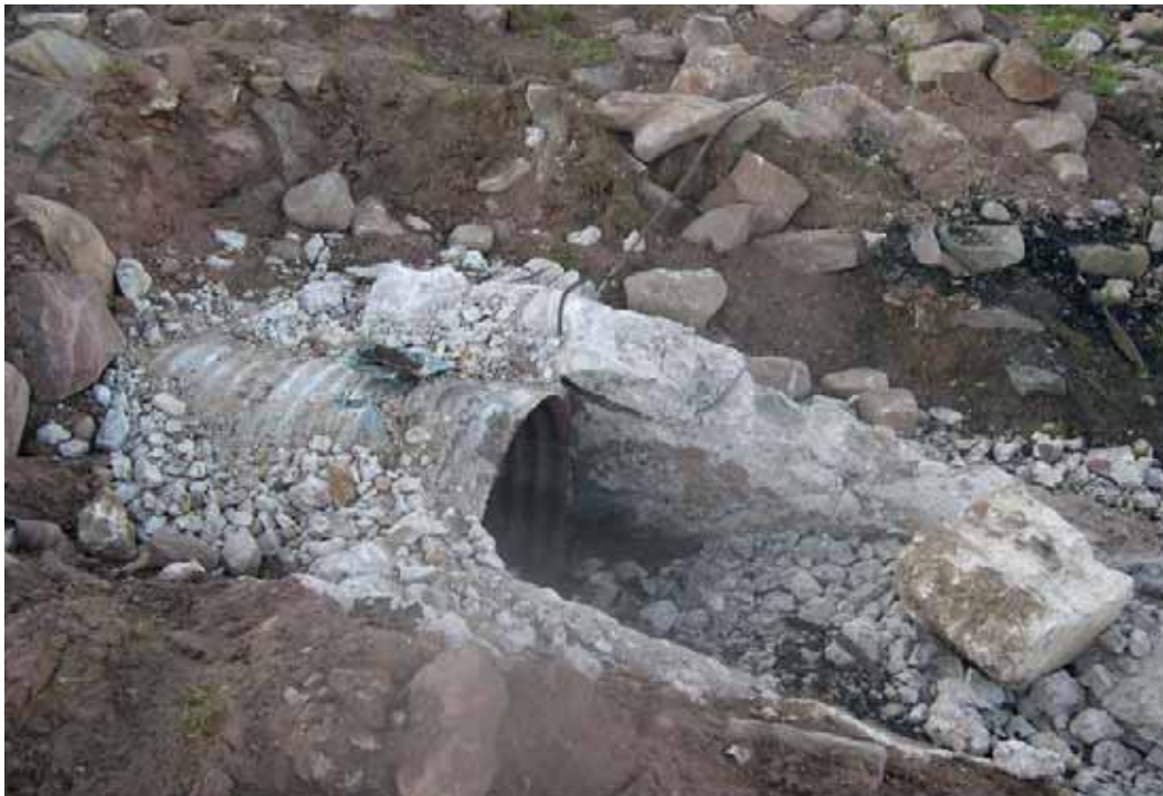
Figure 23 - View of inlet structure prior to backfilling with grout. Demolition was accomplished by heating structure with fire to weaken concrete and using hand tools to break up concrete around the pipe. Demolition performed by SCA crews.
