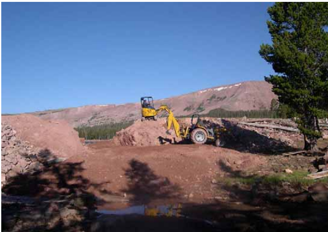
Figure 15 - Initial excavation through the dam. Tractor and mini-excavator are being used for excavation.
