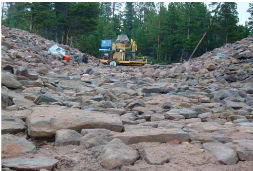
Figure 26 - View looking downstream through the excavated and rip rap lined breach. Note grout plant that was positioned to grout the outlet pipe.
