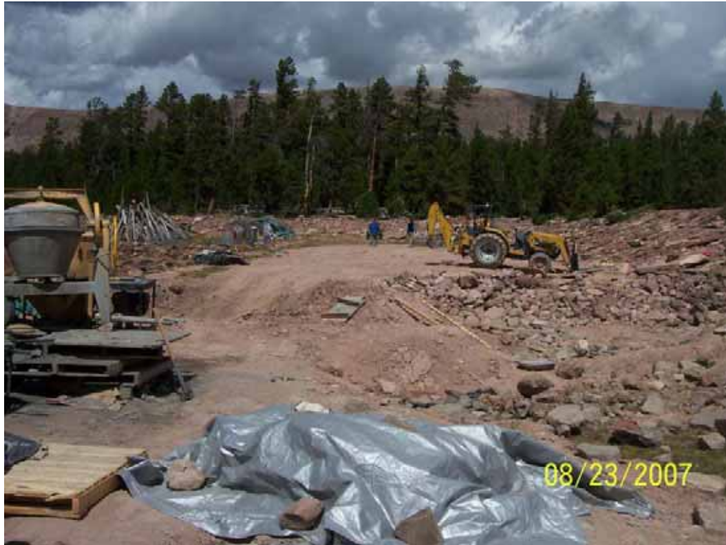
Figure 25 - View of work area during outlet grouting operation. Note inlet channel remaining to be lined with riprap.
