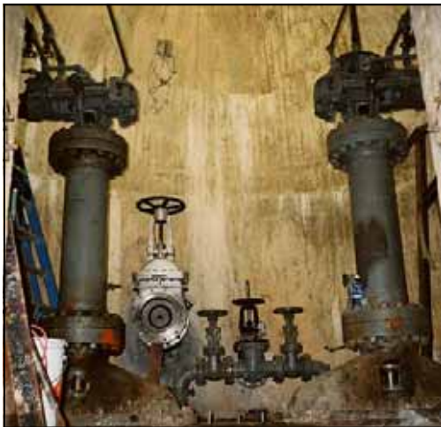
Looking into gate control chamber showing completed valve installation on Moon Lake Dam outlet works. When complete in 2006, this will facilitate release of instream flows from the Dam.
