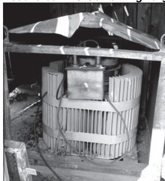
Recovered RTG Containing Large Amounts of Strontium-90
