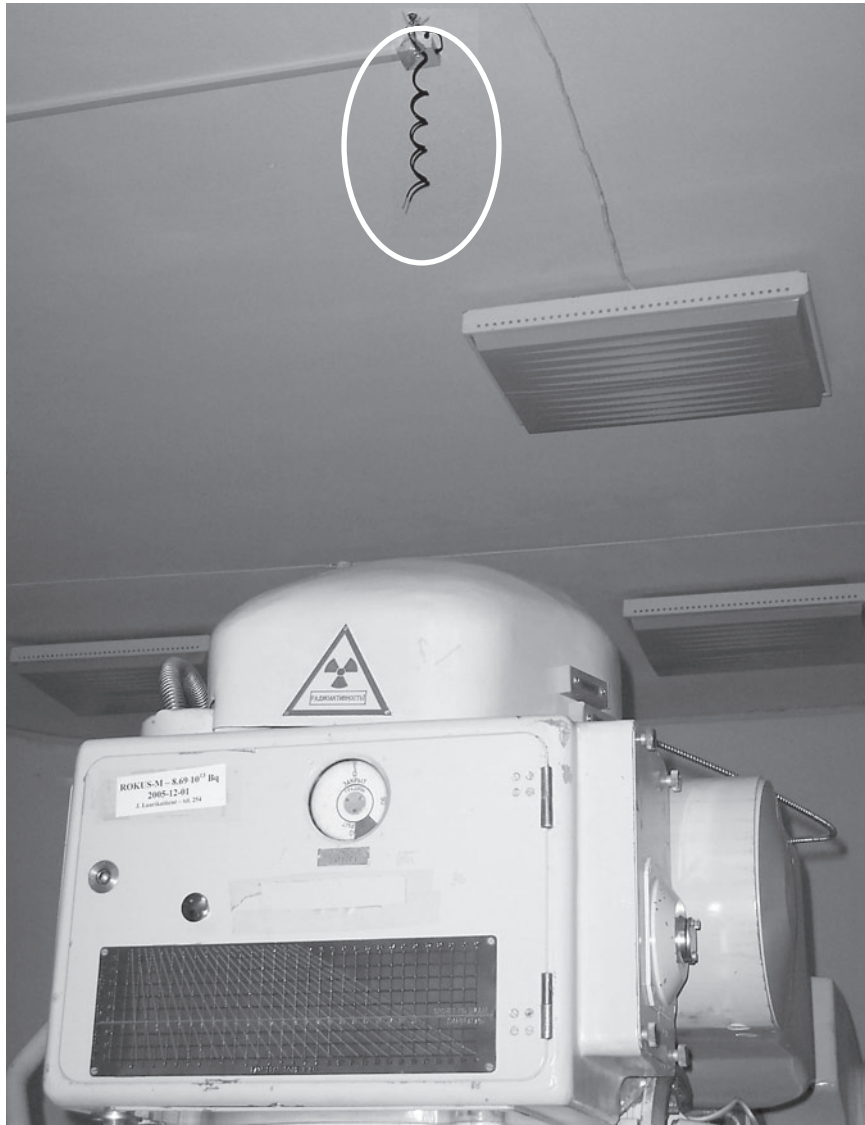
Figure 6: Broken Security Cable at the Oncology Clinic
