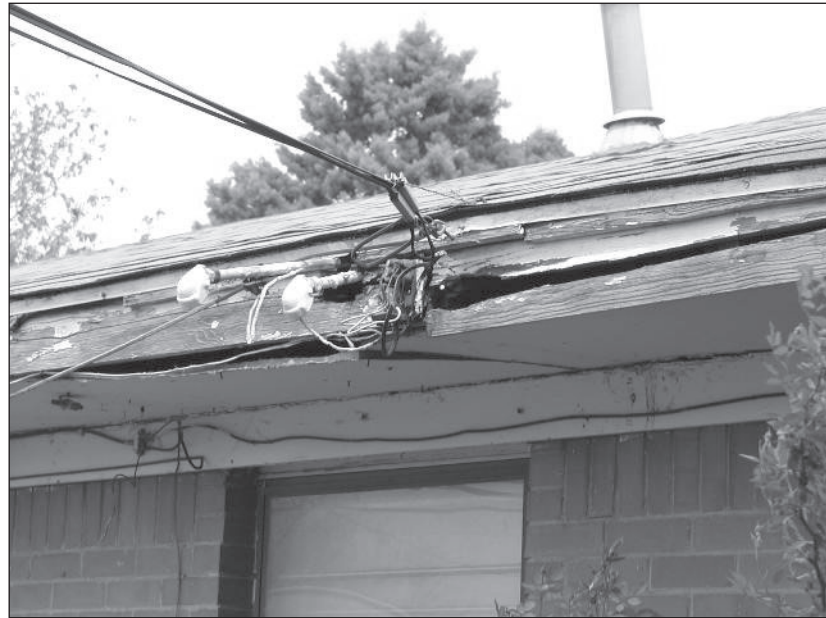
Figure 4: Structural Damage at an Oklahoma Property for Sale
