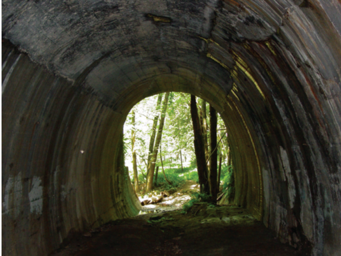
Figure 3-6. View looking out of the west end of Wrights Tunnel toward Los Gatos Creek. The tunnel is now full of leaking cracks that are feeding a small stream flowing from the mouth of the passage.
