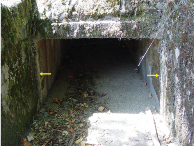
Figure 6-11. This culvert built by Vernon Pick in 1955 displays evidence of right-lateral displacement, possibly from ground motion (creep) along the San Andreas Fault. The arrows on this image show where to look for fractures and offset. Fractures and traces of offset are visible at both ends of the culvert.
