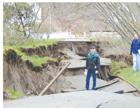
Earthquake damage: engineers examine a lateral-spreading soil failure adjacent to Capitol Lake in Olympia, Washington, after the 2001 Nisqually earthquake. [Photograph by Pedro Arduino, University of Washington.]
