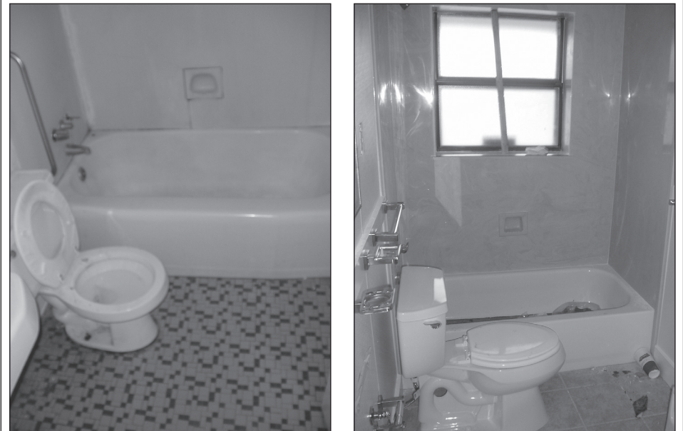
Housing unit with bathroom scheduled for renovation (left) and housing unit with partially renovated bathroom (right).
