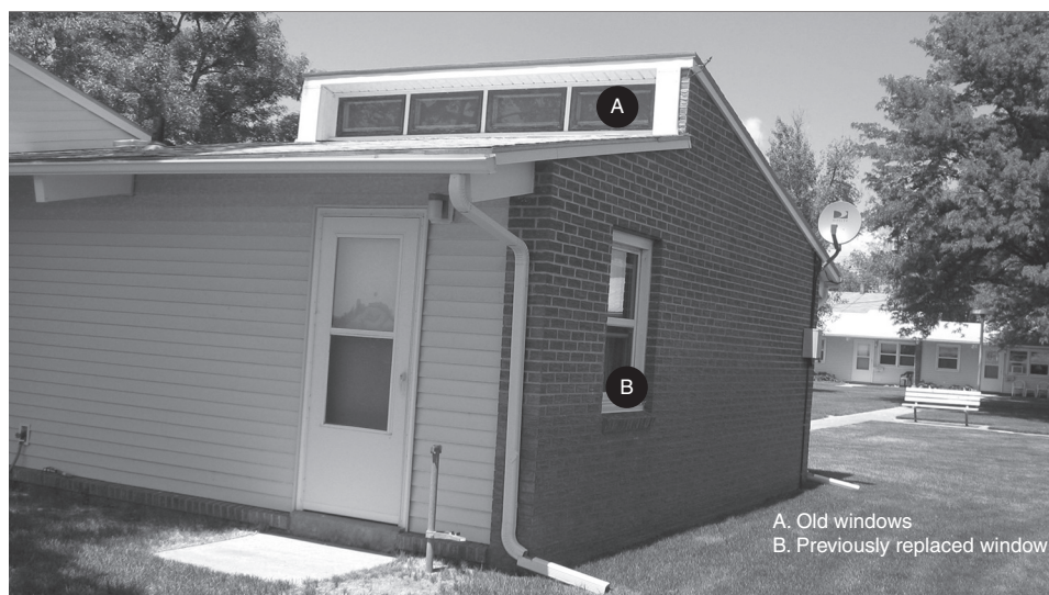
Figure 4: One Public Housing Unit at the Kersey, Colorado Housing Authority Before New Energy-Efficient Windows Were Installed (Upper Windows)
