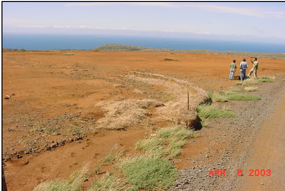
Piligrass bales used to divert water away from road shoulders before causing further damage down stream. Structure was installed in early 2003. Photo taken in April 2003
