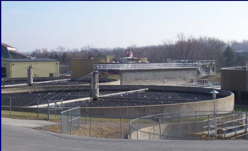
Harold Street wastewater treatment plant
