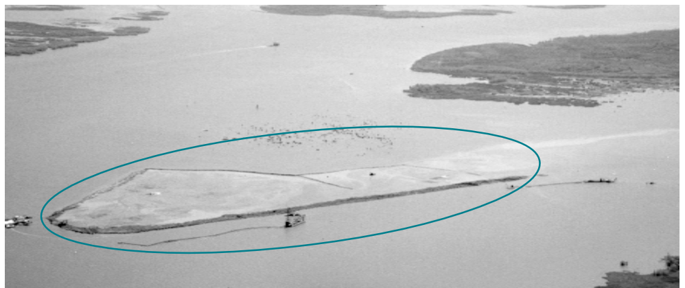
Construction on the first lobe island at Big Island is under way as shown in the photo above. Dredges collect sediment from the surrounding waters and pump it into the island area to build it up. (DNR photo)
