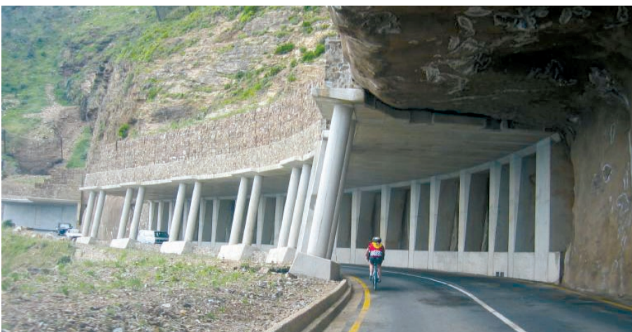
Figure C27. Example of a reinforced rock ledge, Chapmans Peak Drive, Cape Town, South Africa. Photograph attribution: http://commons.wikimedia.org/wiki/Image:Chapmans_peak_dr.jpg .
