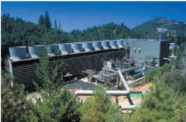
Clean, baseload, distributed electricity is being produced from geothermal resources today. Big Geysers, a 75-MW geothermal power plant located in northern California, is shown above.
