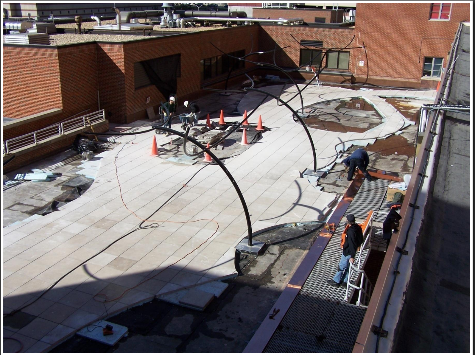
A concrete saw was then used to cut the tiles forming the plant beds
