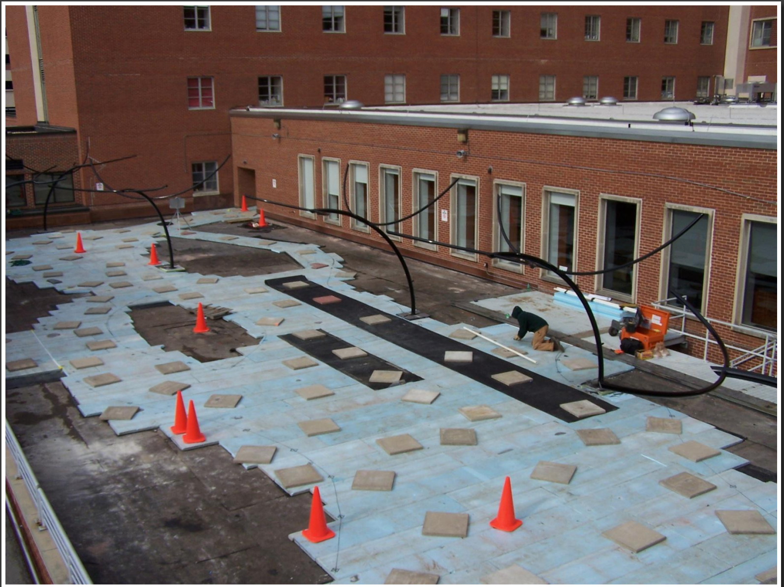
One worker then laid out the pattern that would be used to cut the concrete tiles and insulation from.
