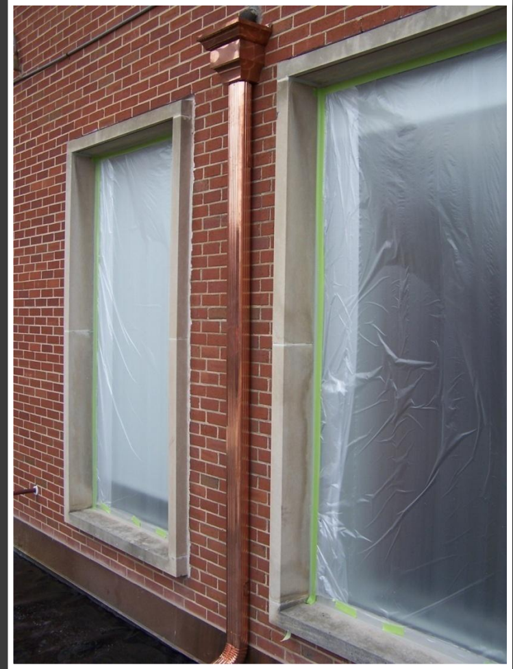
Nice copper downspouts were installed to direct water from the flower box to the terrace.
