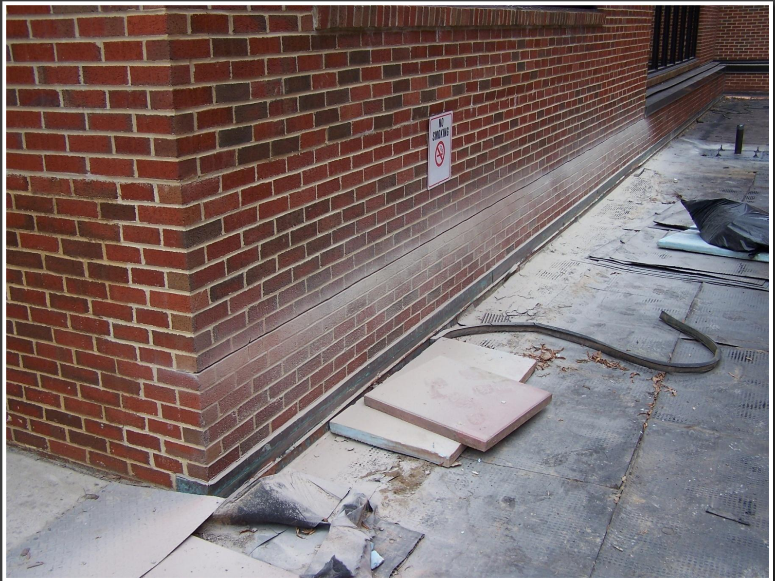
A concrete saw was used to create a lip for the new copper lining that was used to protect the wall and roof from water and soil.
