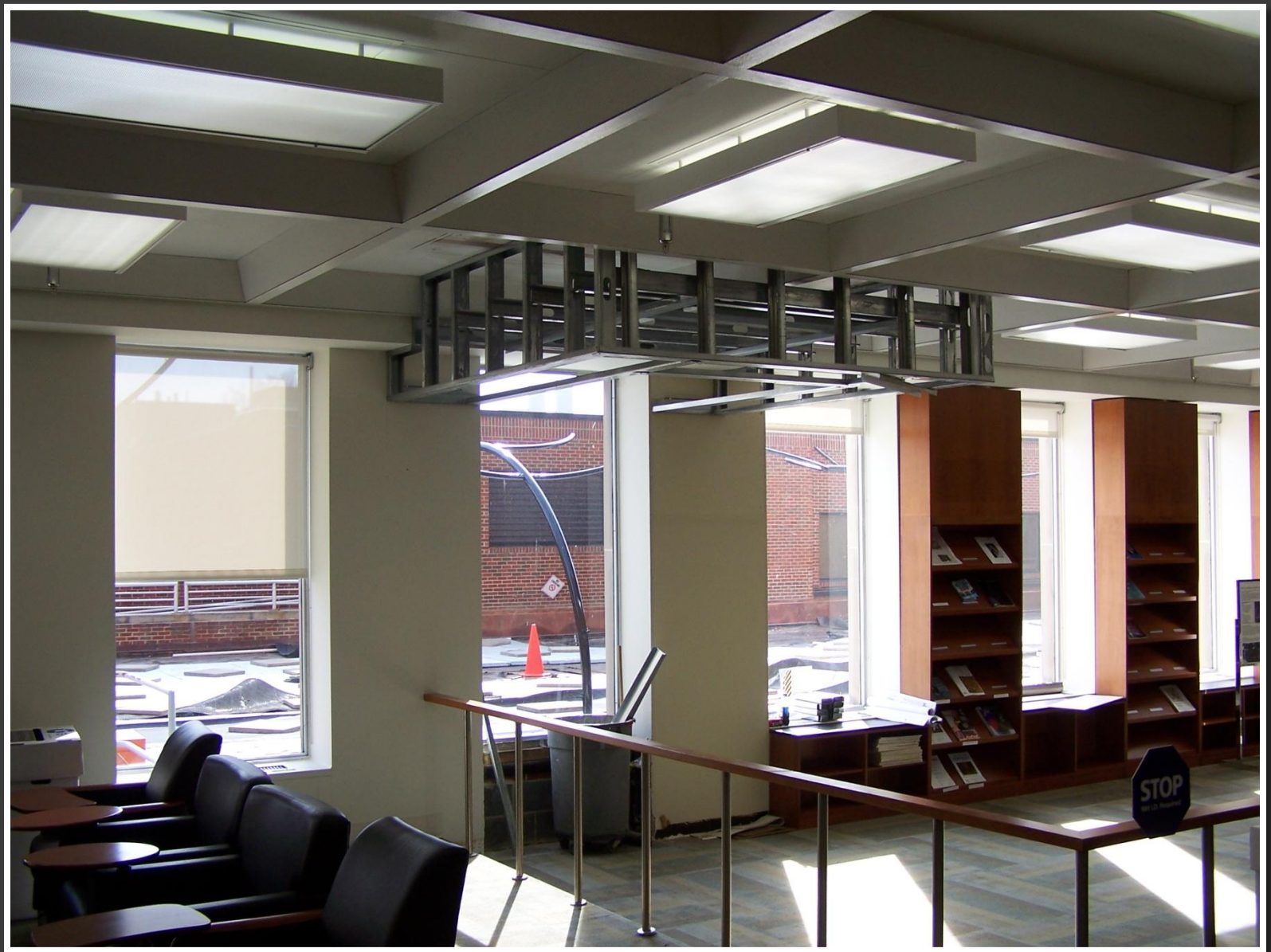
At this time, work began on the vestibule that would become the entrance to the patio from the Library reading room.
