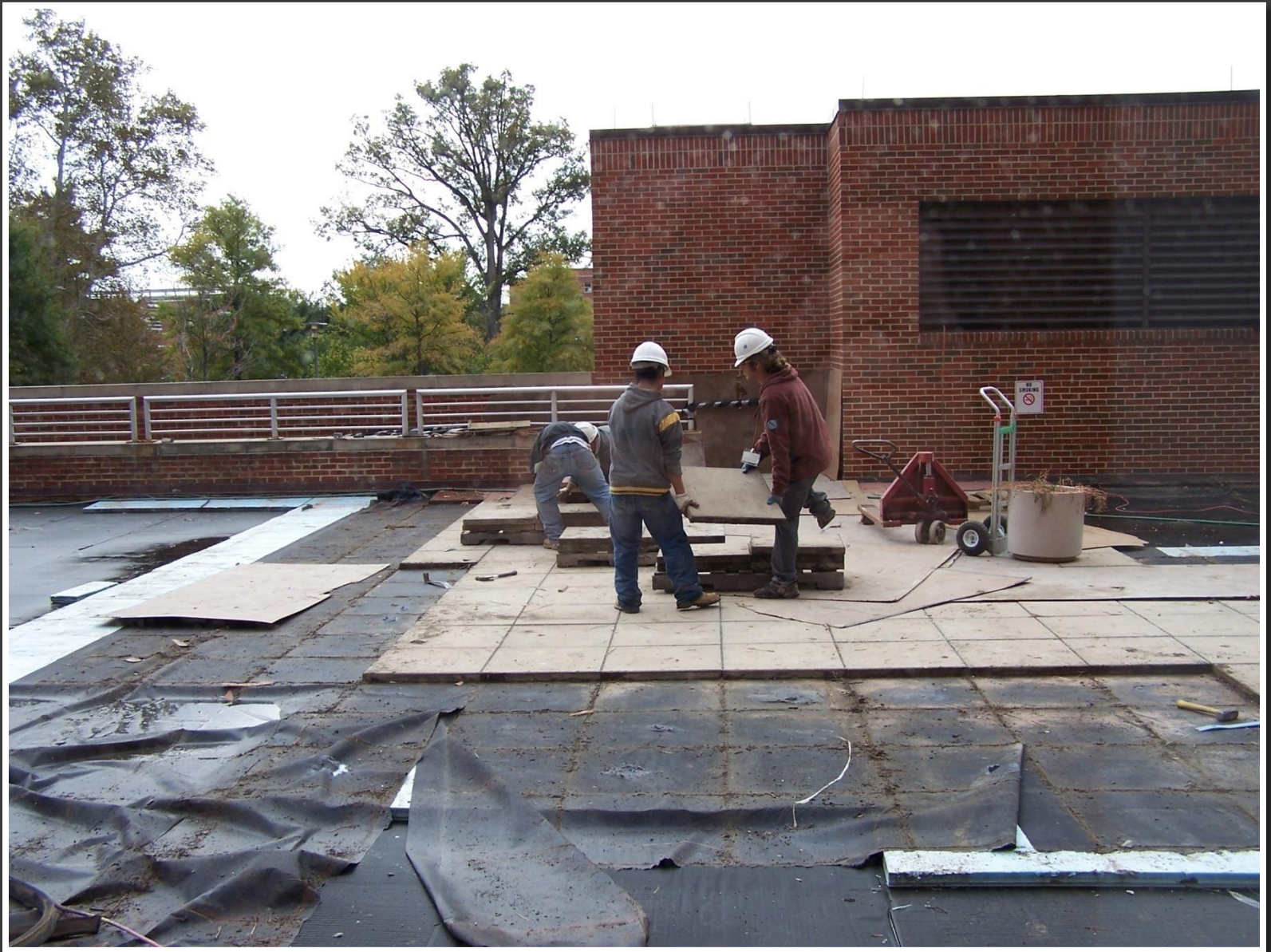
Workers hand carried each concrete tile onto pallets and transported them to a staging area on the outskirts of campus.
