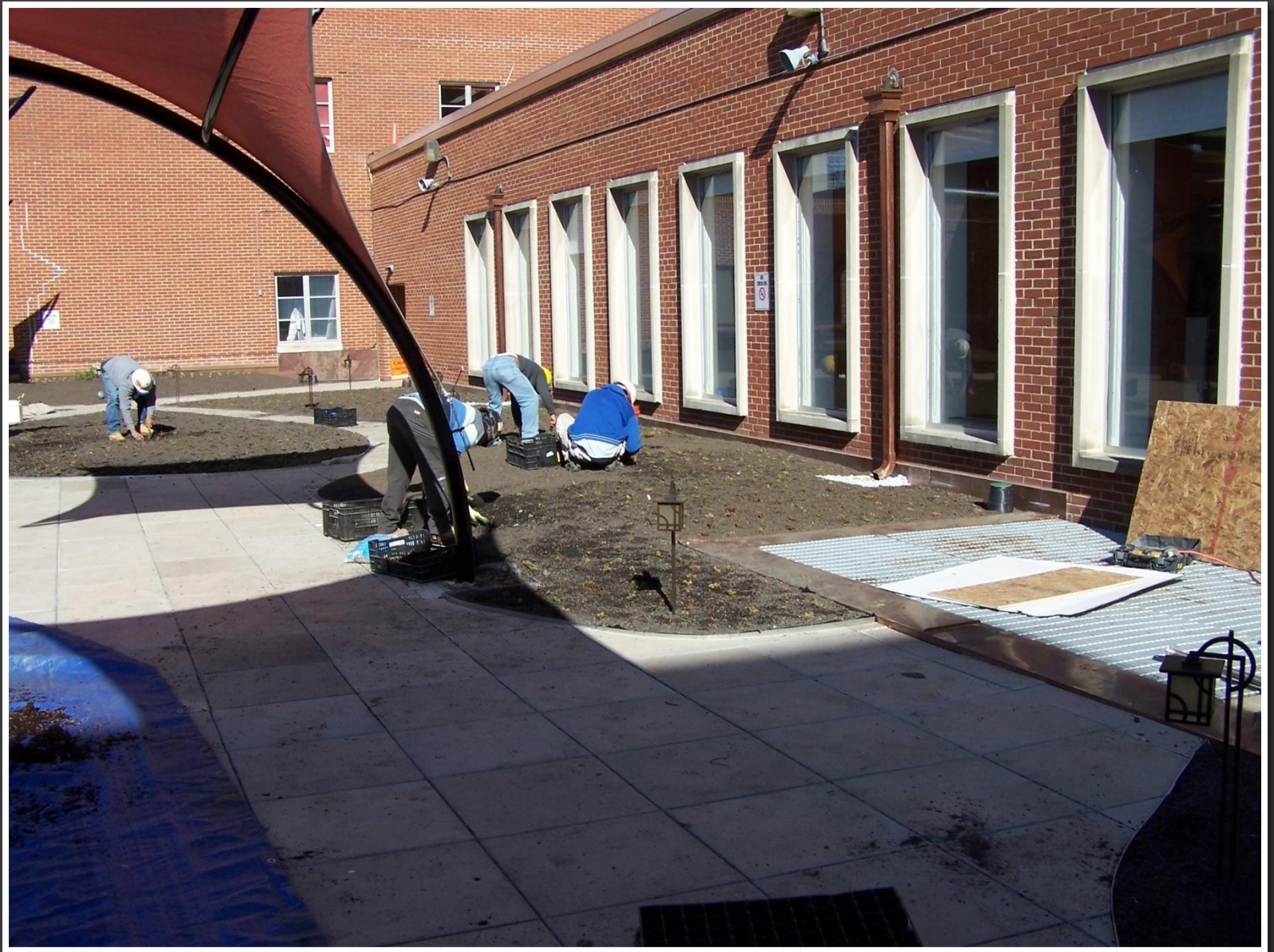
With only three days left until the Grand Opening workers began to install the green roof plants.
