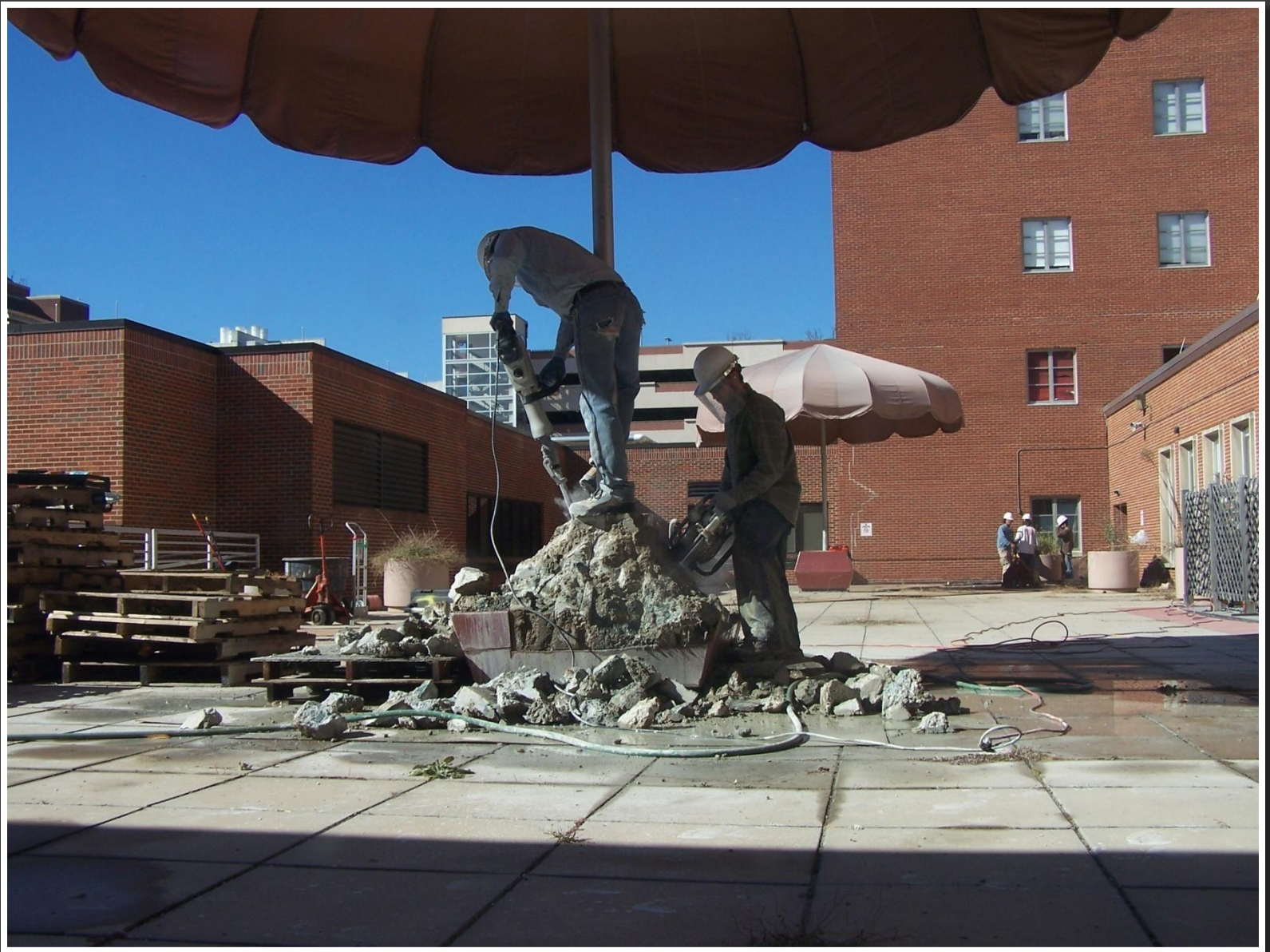
De-construction began in 2008 with the removal of the umbrellas. The stands were constructed of solid concrete that took days to remove.
