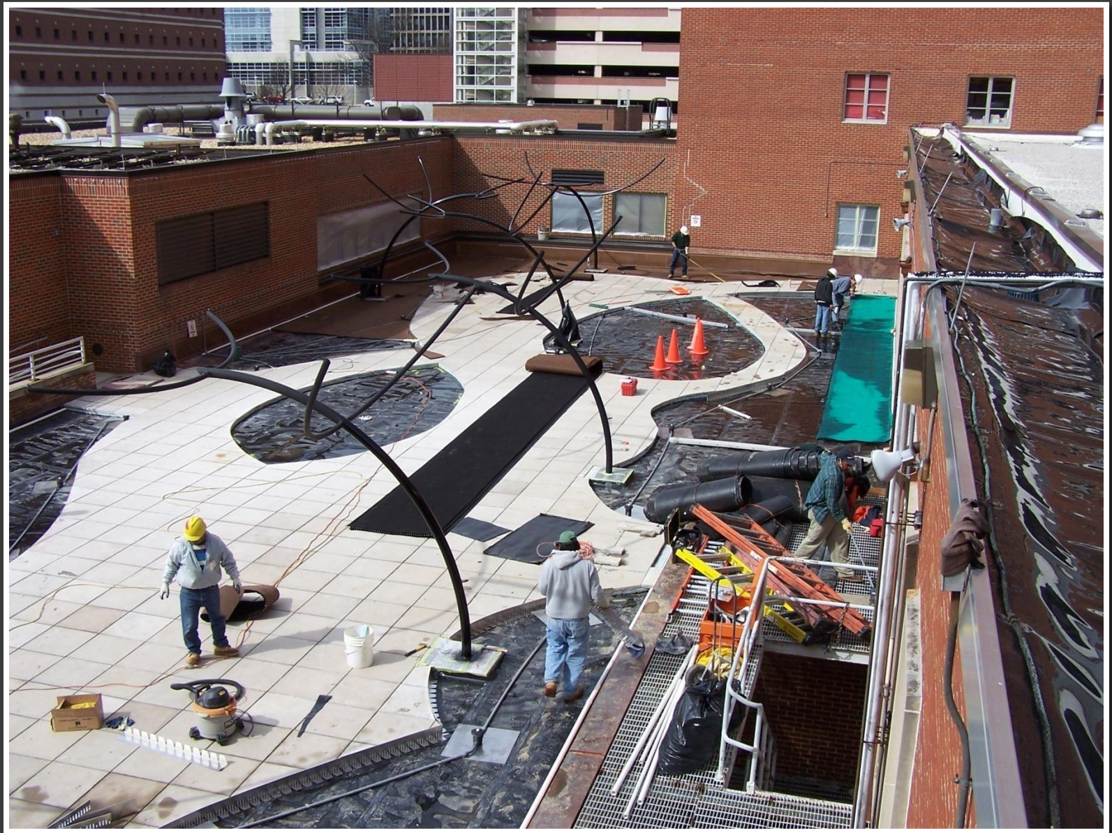
Here workers are laying out additional layers of green roof materials. Note the flower box to the right of this picture with its protective barrier.
