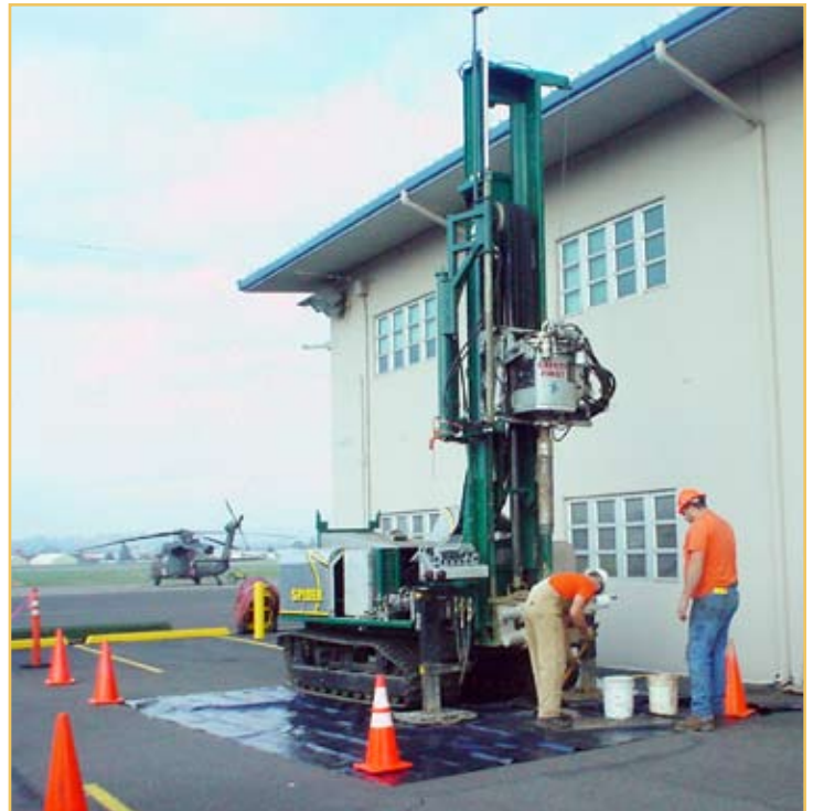
Drilling contractors installing groundwater monitoring well for vapor intrusion assessment use a limited access sonic drilling rig adjacent to active flight line at Army Aviation Support Facility #1.
