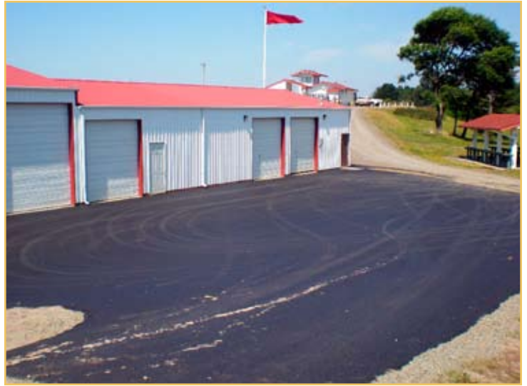
Completed engineered cap over former landfill at MARF Range Maintenance Building, Camp Rilea.
