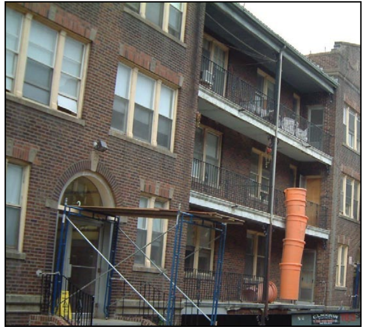
Nazing Apartments, in Roxbury, Massachusetts, is pictured here during the renovation of 144 units of affordable housing. This project received bank financing through the Part 24 Public Welfare Investment Authority.
