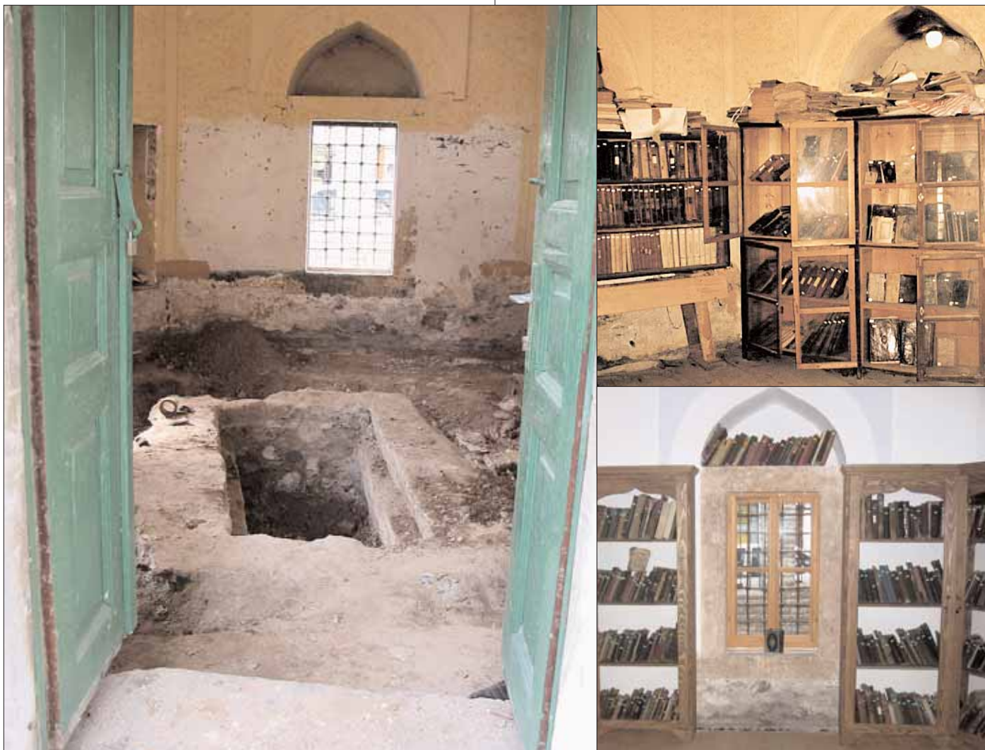
[clockwise from left] Empty tomb chamber discovered during restoration; library before restoration; library after restoration, Gazi Mehmed Pasha Library, Prizren, Kosovo. U.S. Mission Pristina
