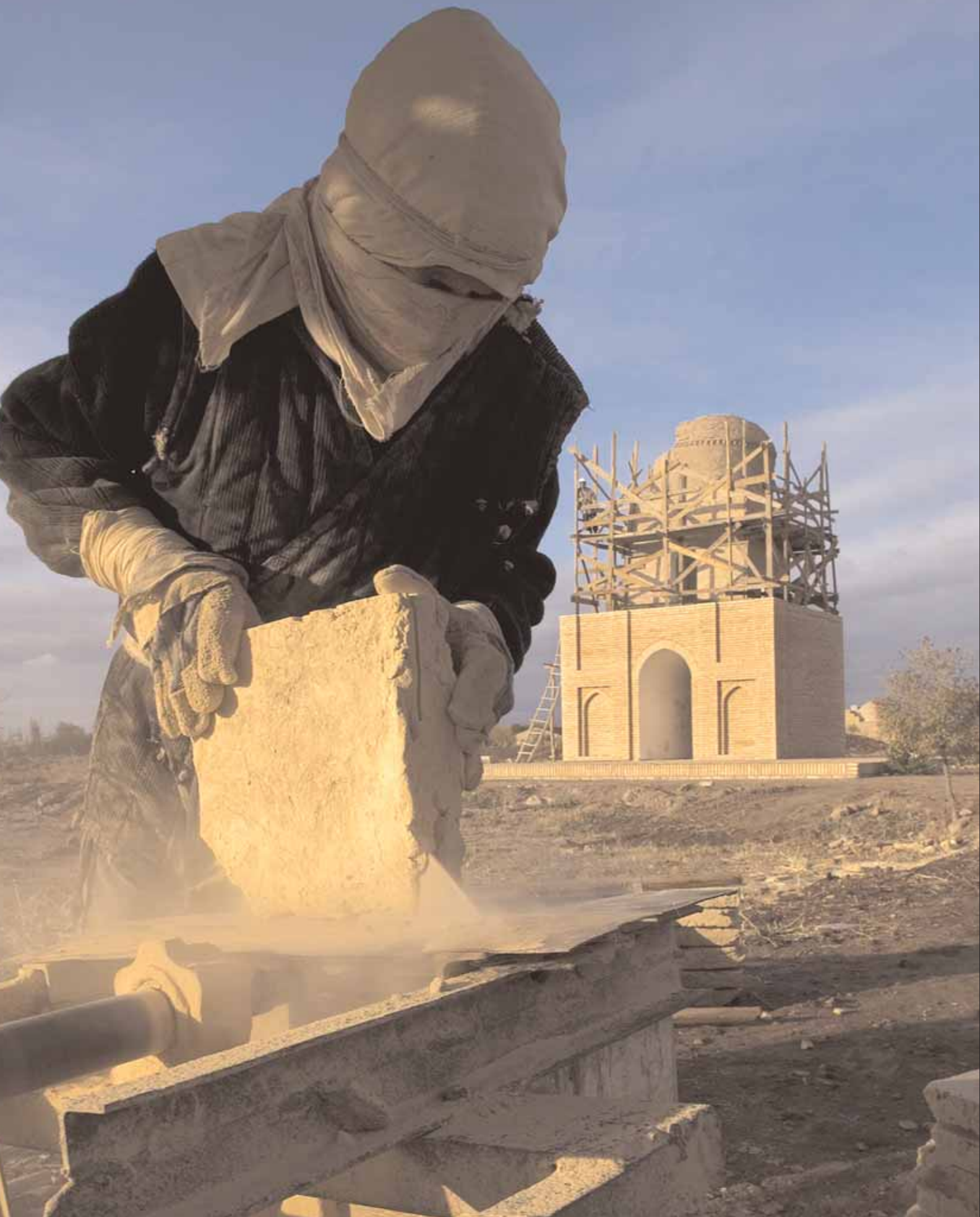
Restoration of Ak Saray Ding Tower, Konya Urgench, Turkmenistan (see page 31). Photograph by Angus McDonald
