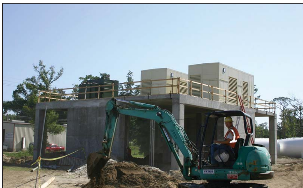
Two generators are in place on an elevated pad located to the north of the main building.
