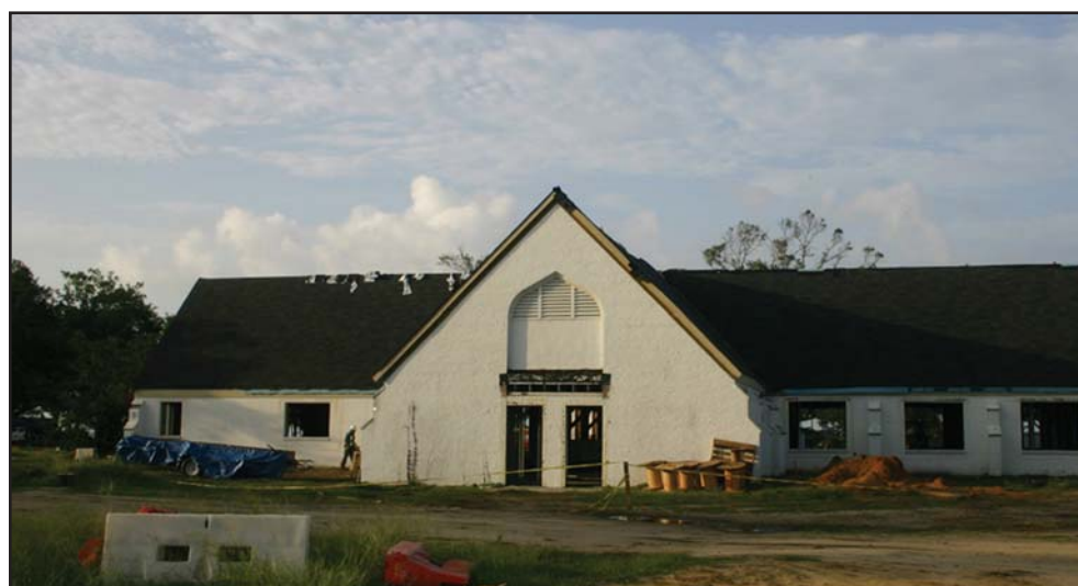
The renovation of the Chapel is underway. This photo shows the new roof on the north side of the building.
