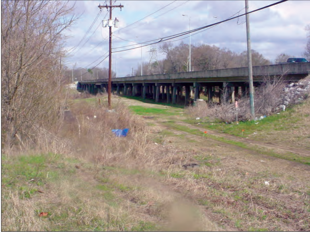
Figure A15. Downstream face of U.S. Highway 31 Bridge, Montgomery, Alabama. (See figure 7 for location.)
