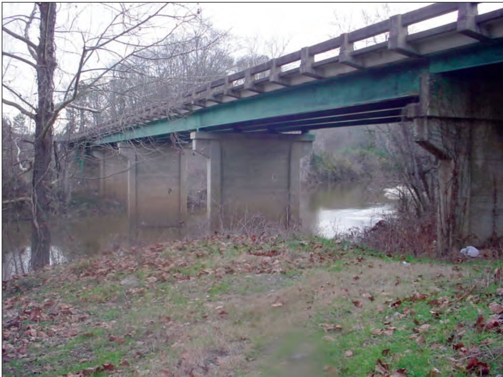
Figure A8. Downstream face of Old Selma Road main-channel bridge, in the vicinity of cross section D, Montgomery, Alabama. (See figures 5 and 7 for location.)
