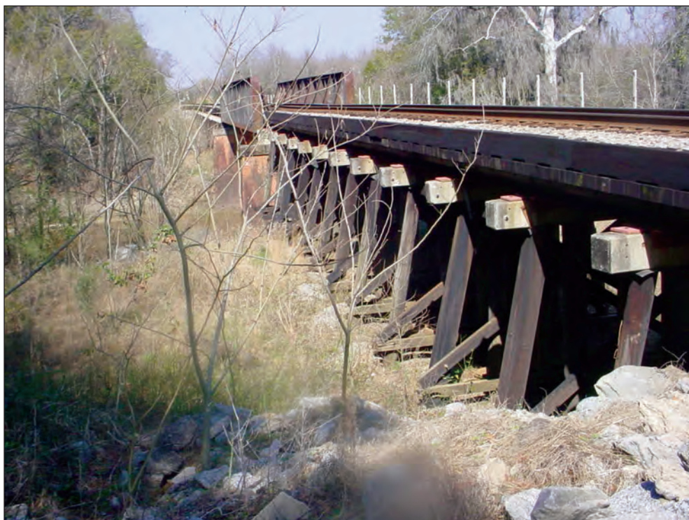
Figure A18. Downstream face of Seaboard Coast Line Railroad bridge, Montgomery, Alabama. (See figure 7 for location.)
