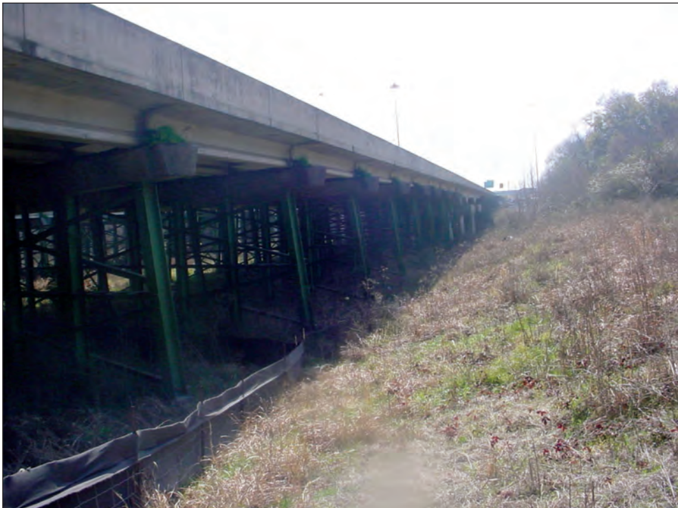
Figure A16. Downstream face of Interstate 65 bridge, Montgomery, Alabama. (See figure 7 for location.)
