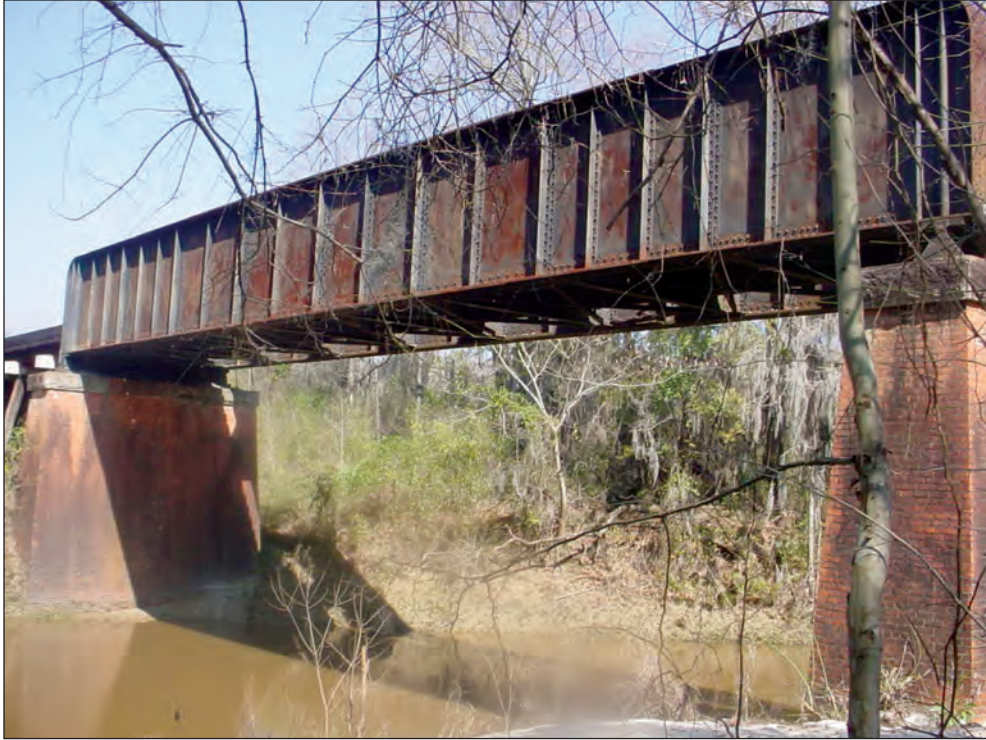
Figure A19. Seaboard Coast Line Railroad bridge, Montgomery, Alabama. (See figure 7 for location.)
