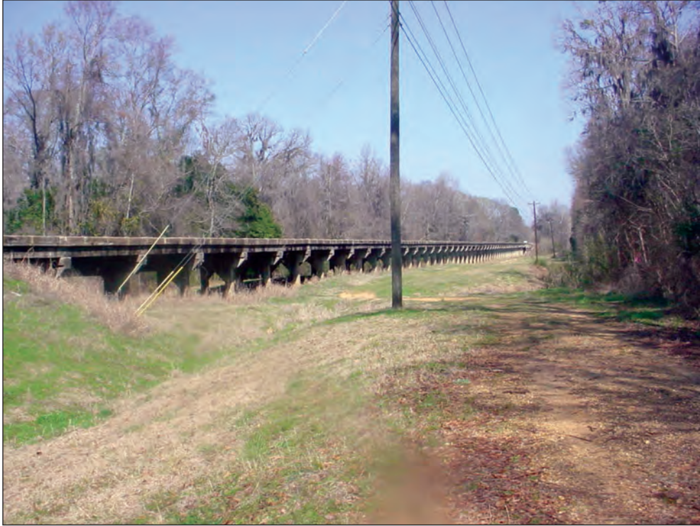
Figure A23. Upstream face of Norman Bridge Road crossing, Montgomery, Alabama. (See figure 7 for location.)
