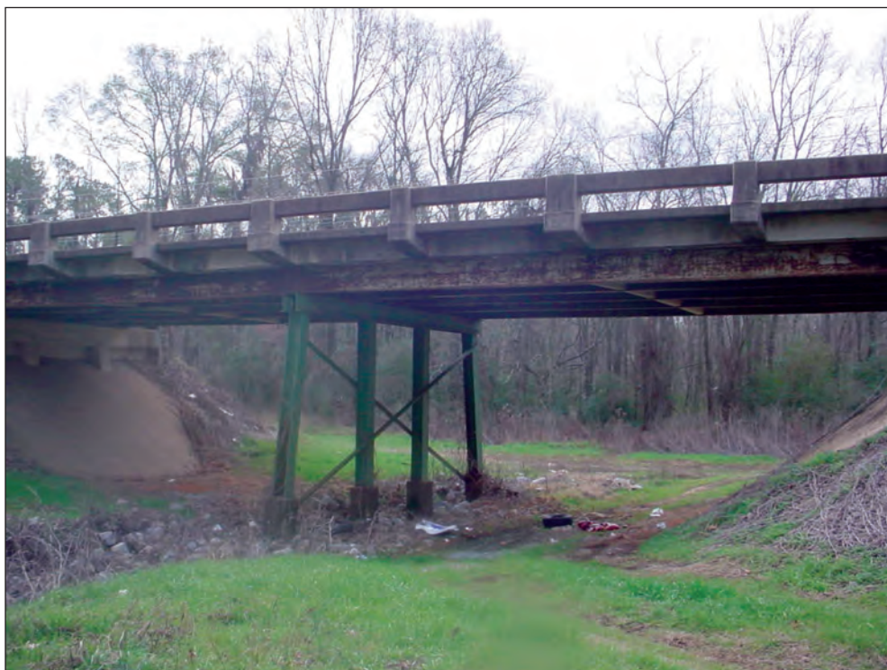
Figure A6. Downstream face of Old Selma Road relief bridge #1, in the vicinity of cross section D, Montgomery, Alabama. (See figures 5 and 7 for location.)
