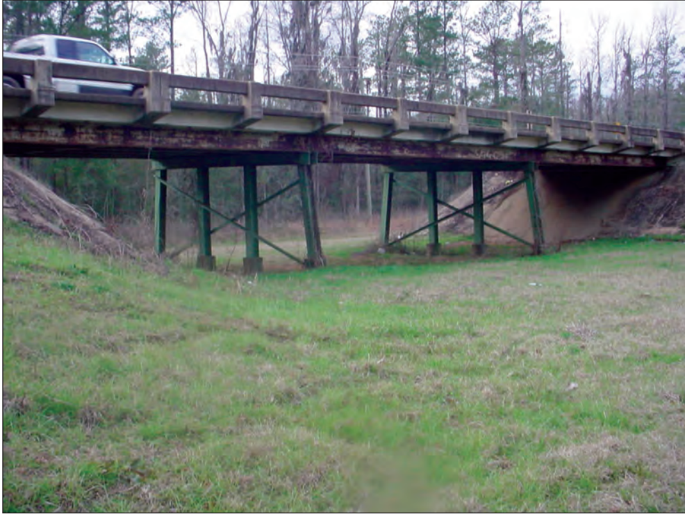
Figure A7. Downstream face of Old Selma Road relief bridge #2, in the vicinity of cross section D, Montgomery, Alabama. (See figures 5 and 7 for location.)
