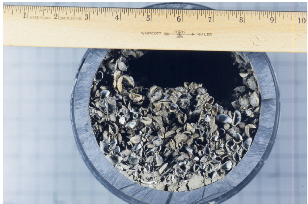
Figure 3-5 Zebra mussels clogging water pipe (USACE photo)
