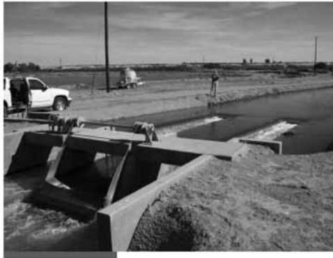
Yuma Water Users Association installed extensive improvements including automated water tracking systems, measurement stations, and key canal structures. Source: U.S. Dept. of Interior website
