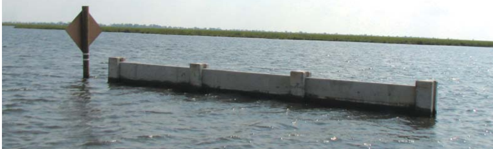
Where bayou bottoms proved too soft to support rock dikes, BA-97 installed test sections of concrete wall. Consisting of panels supported by pilings sunk deep in the mud, such structures offer more stable protection.
