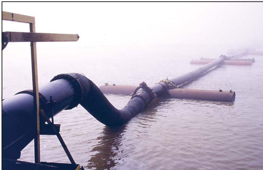
In the Atchafalaya Sediment Delivery Project, dredged sediments were pumped through a pipeline toward the marsh creation disposal area.
