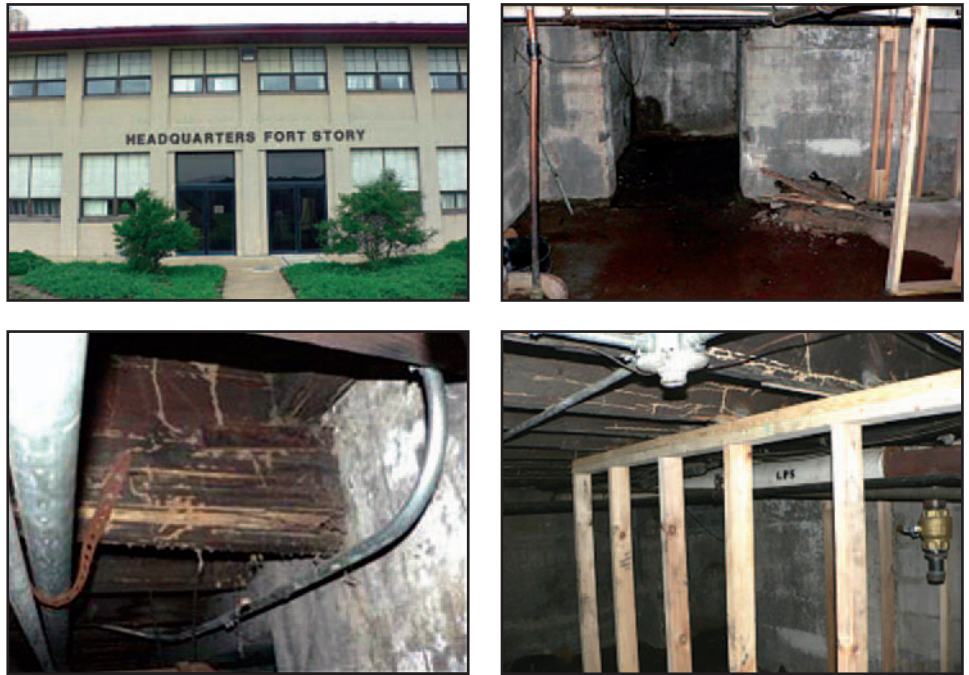
Figure 2: Damaged Basement in the Command Headquarters Building at Fort Story
