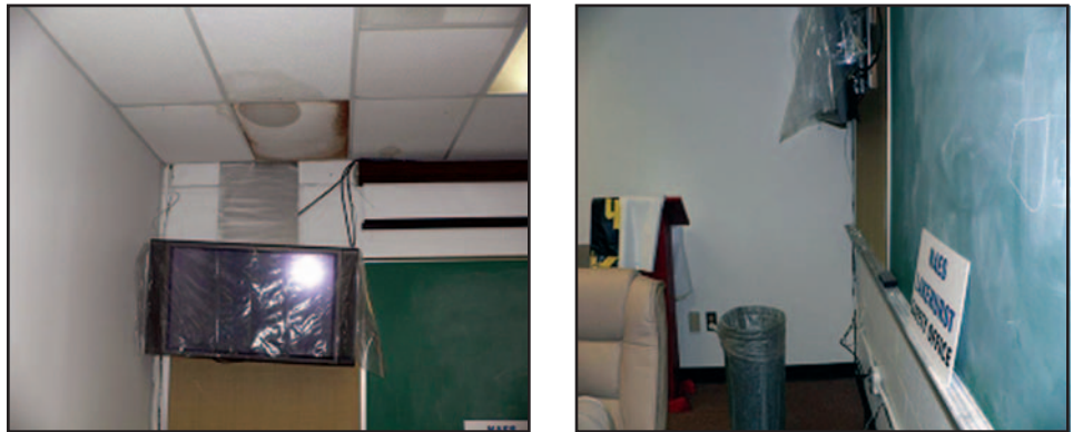
Figure 5: Damage from a Leaking Roof at the Public Works Building at Naval Air Engineering Station Lakehurst
