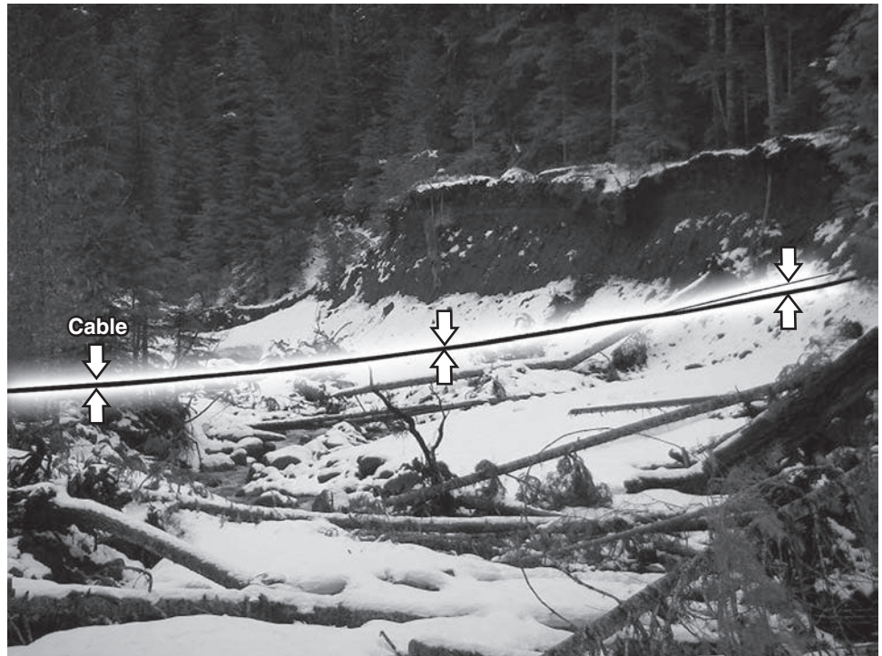
Figure 5: Exposed, Hanging Cable at Mount Rainier National Park
