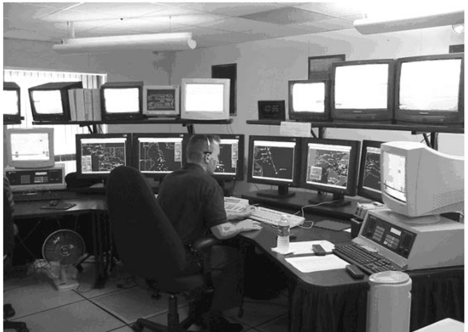
Figure 1: Staffed VTS Control Room, Houston, Texas
